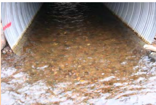
Outlet of Pipe
