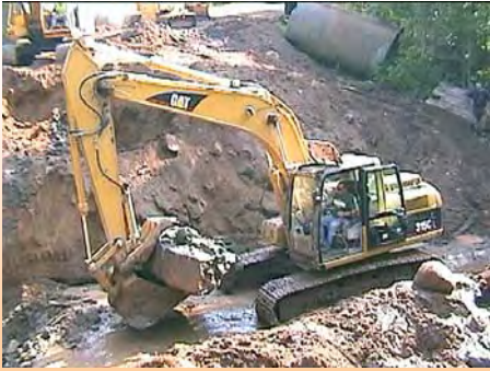
Massive Pieces of Concrete Buried at Site
