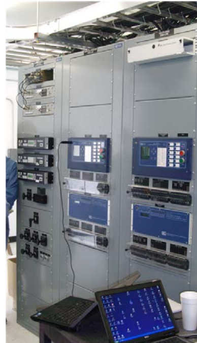
Knoll Substation control house with PMUs and PDC
