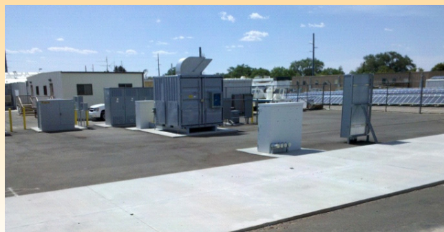
The Energy Storage Test Pad.
