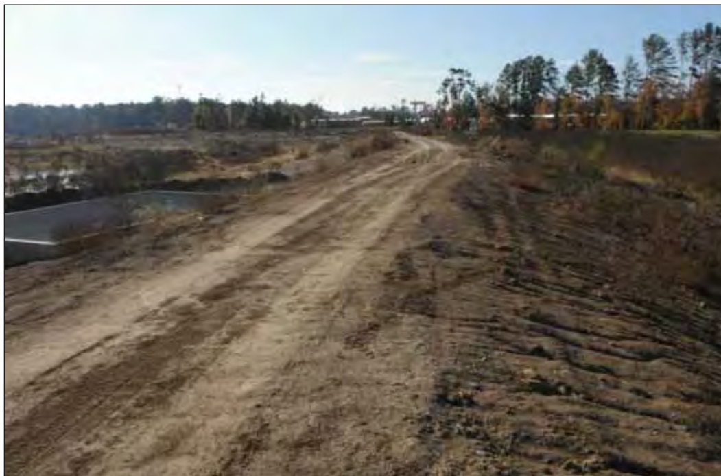
Figure 12. Access Road, Storm Water Drain, and Detention Pond under Construction in Western Portion of APE (Facing S)
