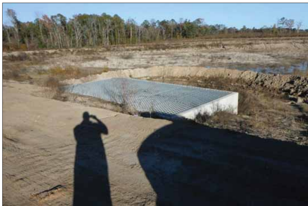
Figure 13. Detention Pond and Storm Drain/Culvert in Western Portion of APE (Facing NE)
