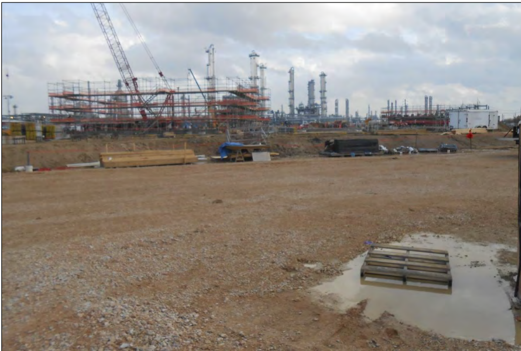
Figure 7. Overview of Existing Fractionator Plant in 58-acre Portion of APE (Facing SE)
