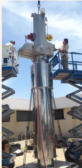
Workers in Jamaica load HEU into the transportation cask for return to the U.S. – Photo courtesy of NNSA.
