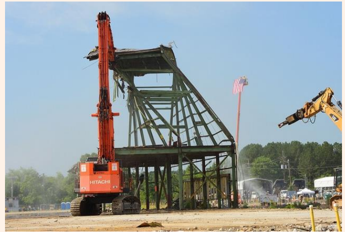
Workers take down the last section of the K-31 building at Oak Ridge's East Tennessee Technology Park.
