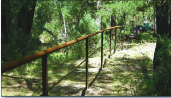
Figure 2. SFNF staff installed this steel pipe fence to prevent ATVs from accessing and damaging the riparian corridor in a recreation area.
