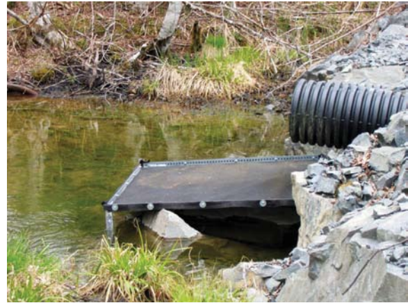
Figure 3. Experimental retrofit for culvert discharge to improve capture of sediment before it enters Granite Creek.
