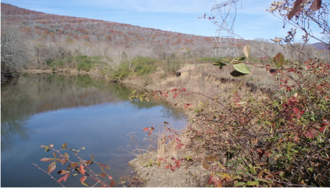
Paint Rock River, AL: Before project: Steep, eroding bank with signs of bank sloughing.
