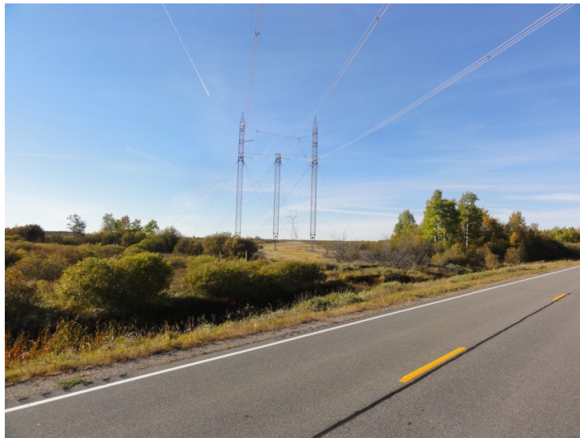
Figure 6.10-3. View of Existing 500kV Transmission Line and Corner Structure at Highway Crossing
