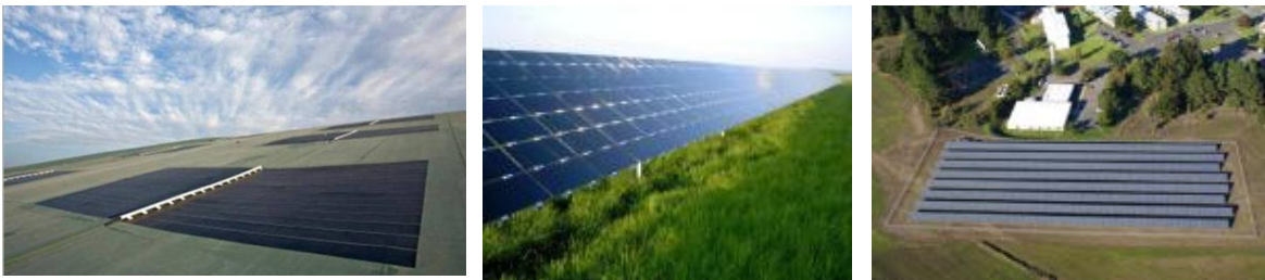
Figure 4. Thin-film solar panels installed on solar energy cover (left) and fixed-tilt mounting system (middle and right). Photos from (left) Republic Services, NREL 23817, (middle) Beck Energy, NREL 14726, and (right) U.S. Coast Guard Petaluma Site, NREL 17395
