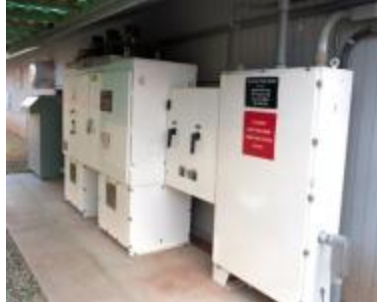
Figure 5. String inverter. Photo by Warren Gretz, NREL 07985
