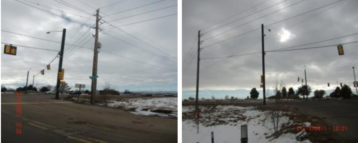
Figure 9. Electrical distribution on the southwest corner of the site at the intersection of North Tower Road and East 6 th Avenue. Photo by Randolph Hunsberger, NREL
