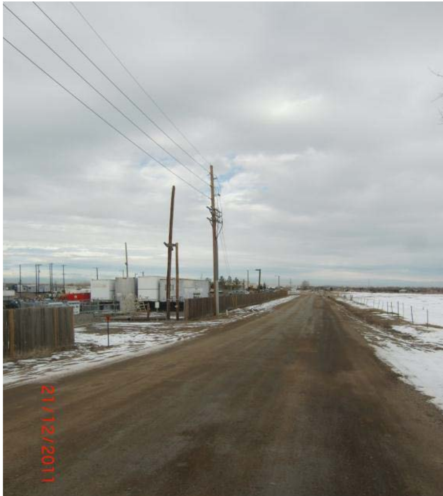
Figure 10. Electrical distribution along the southwest side of the site along North Tower Road and the possible electrical tie-in point for the PV system at the Tower Road site. Photo by Randolph Hunsberger, NREL
