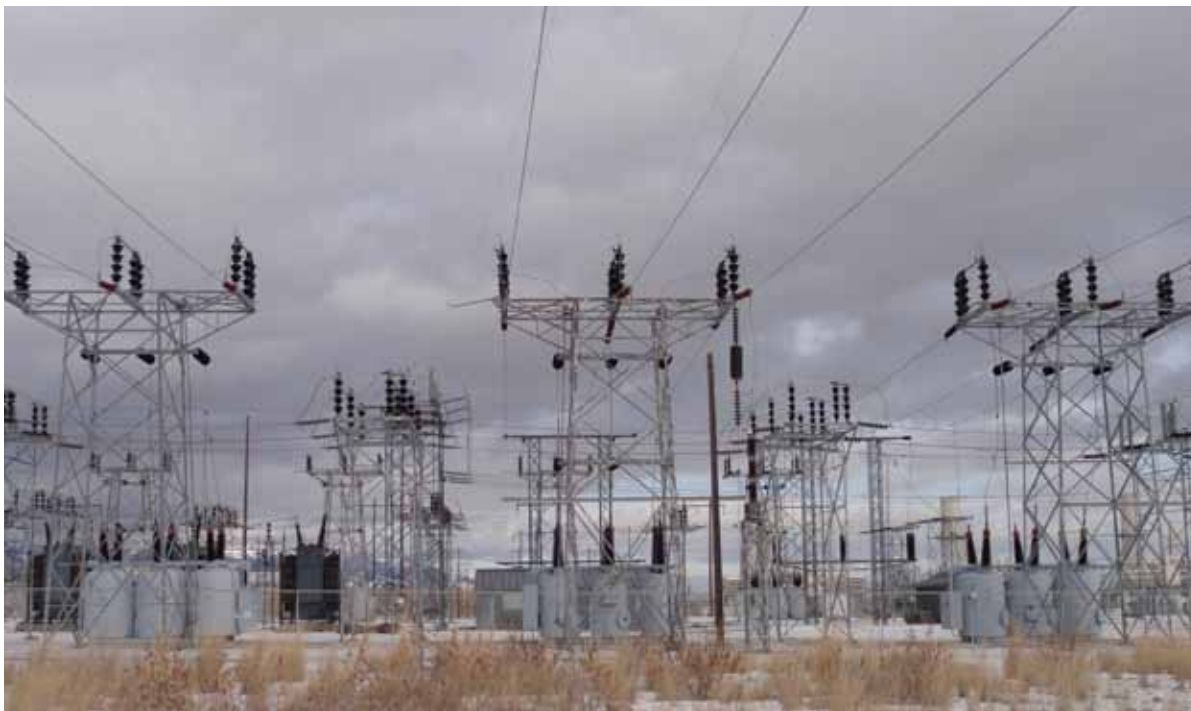
Mill Creek Substation, Anaconda, MT
