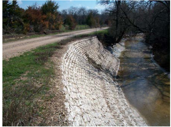
Figure 2 – Streambank Protection: Stacked concrete bags
