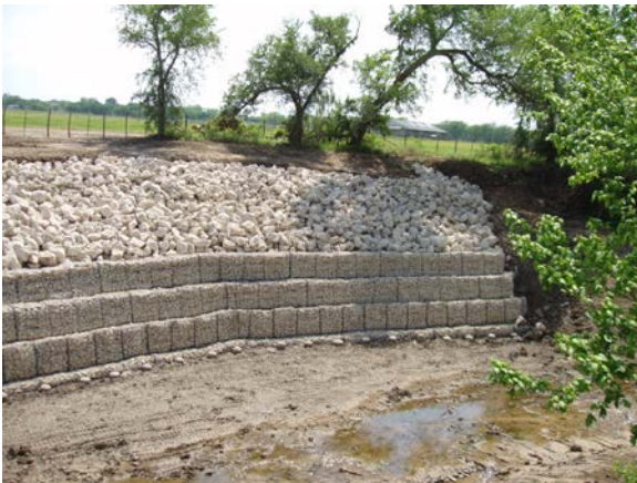
Figure 5 – Streambank Protection: Gabion Baskets with rock armor.
