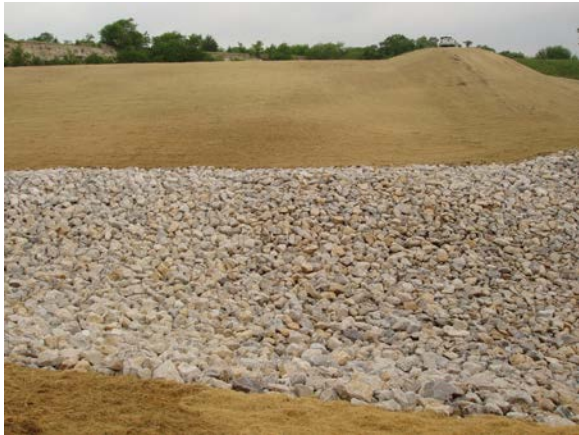
Figure 14 – Flood Retarding Structure: Earthfill, shaping and rock armor at outlet of auxiliary spillway.
