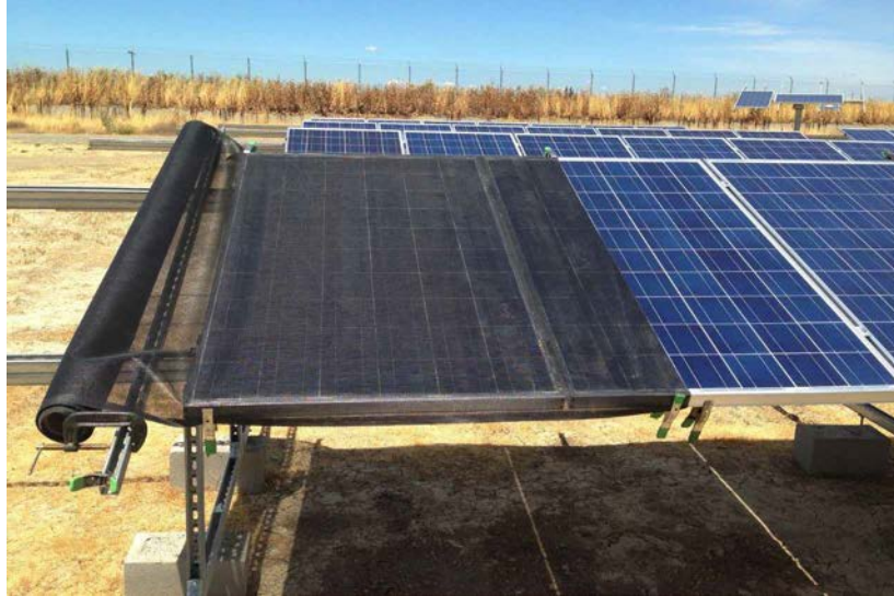
Figure 7. Close-up view of shading mesh on a single string.
