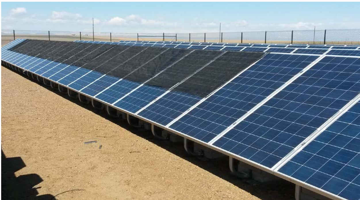
Figure 12: Maxim installation at the Aurora, CO, site (Unshaded panels in the foreground are not included in the partial-shade experiment).
