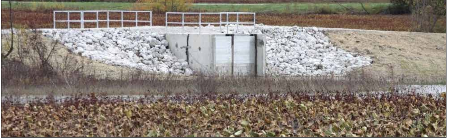
A water structure at Pool 2B can be open and closed, allowing for fish to move through. USFWS
