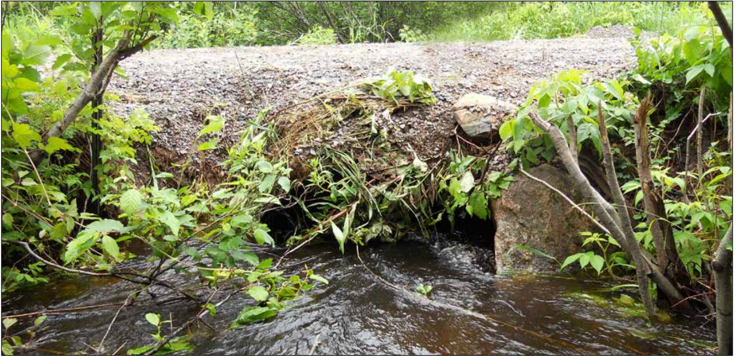
Structural barriers like culverts act as barriers to fish passage. This culvert was replaced in Norman Creek River in upper Wisconsin. USFWS
