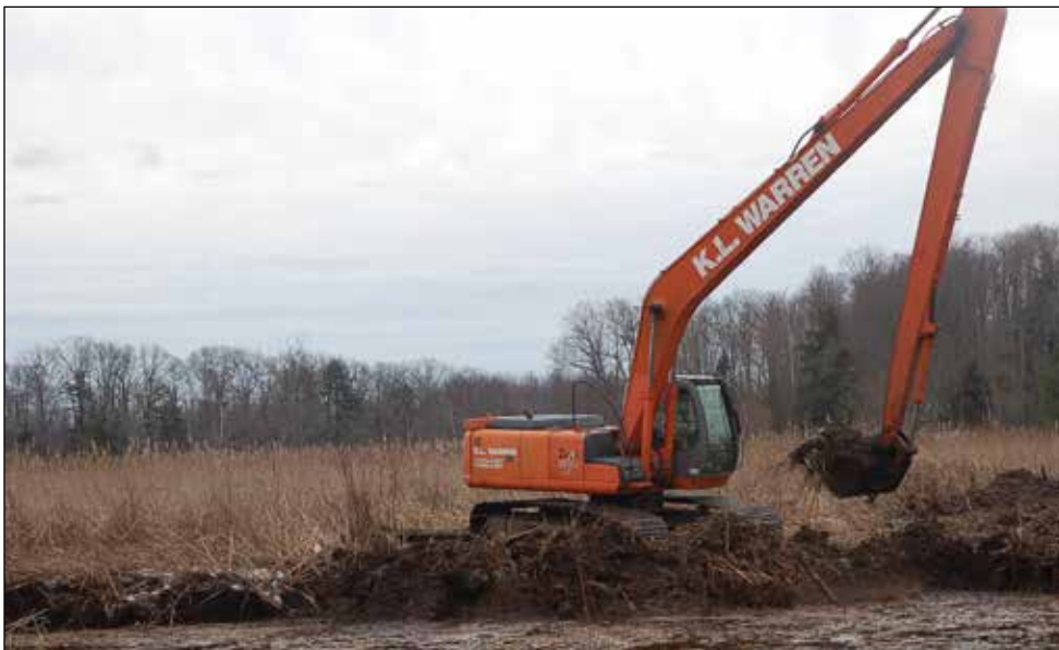
Photos, from top: Digging a new stream channel at Lakeshore Marshes Wildlife Management Area. Post restoration efforts at Lakeshore MWMA. Creating pothole habitat at Lakeshore MWMA. All photos USFWS
