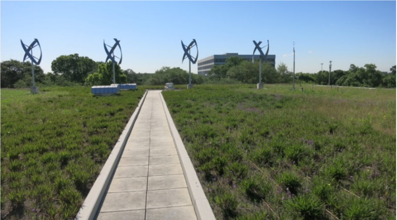
Figure 12. NASA Building 12 wind turbine installations. Photo by Dave Jager, NREL
