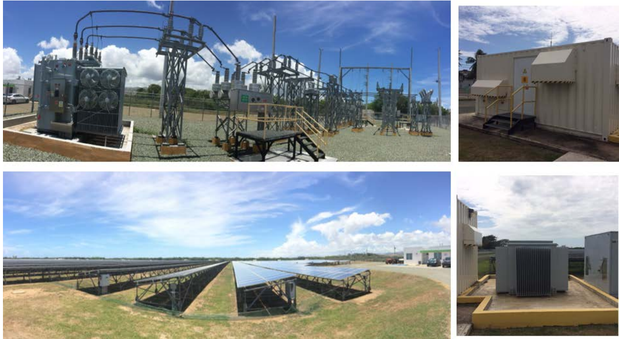
Figure 16. Photos of Ilumina PV power plant substation and PV array. Image from NREL
