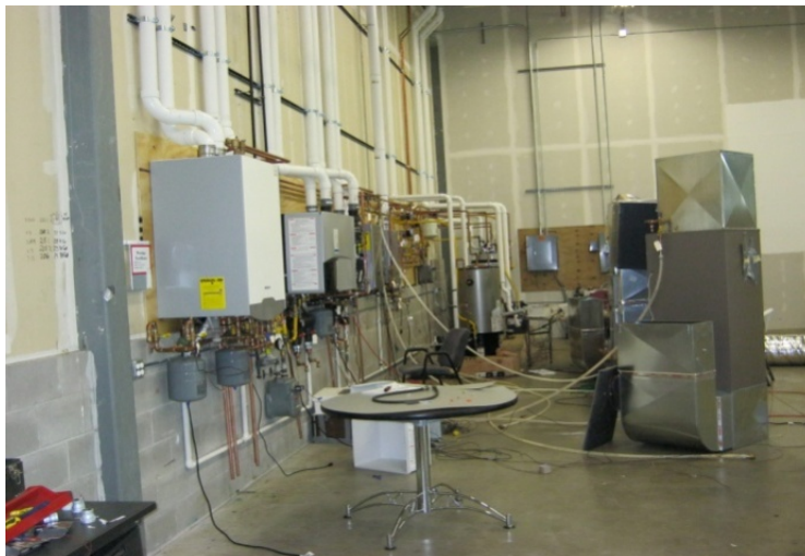
Figure 15. Integrated space and water heating test laboratory
