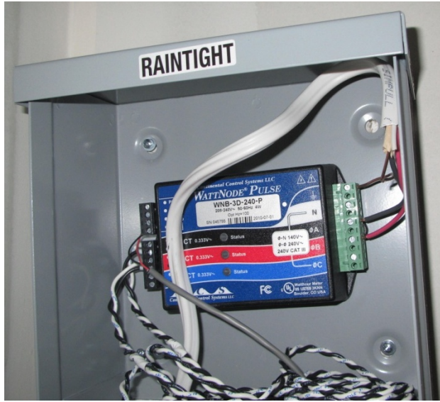
Figure 25. The wires from the CTs and the voltage tap are connected to the WattNode Watt-hour transducer.
