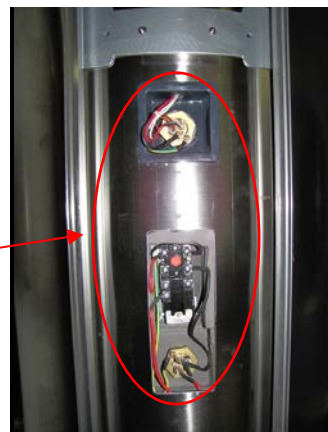
Figure 12. Both heater covers removed. The upper heater is the main heater and the lower heater is the backup (not connected).
