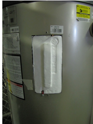
Figure 9. The Styrofoam insulation that covers the upper heater access point.
