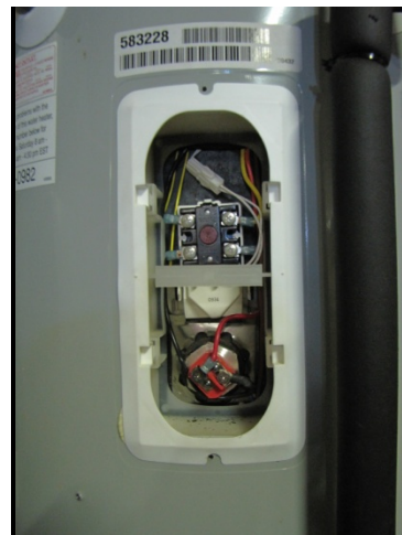
Figure 7. After the insulation is removed, the tank wall is accessible for installing a TC.
