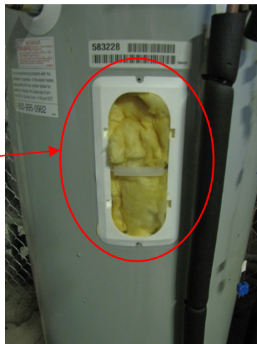
Figure 6. The top heater access point with the cover removed. The fiberglass insulation can be removed.
