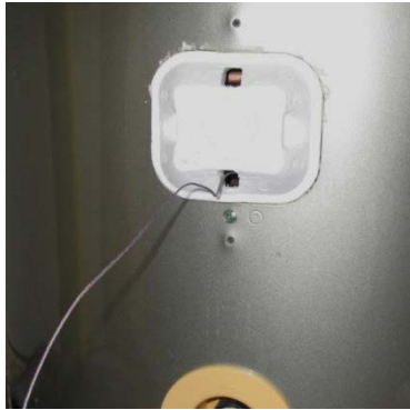
Figure 3. The insulation is replaced and the TC wire is directed through a hole in the insulation.
