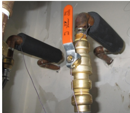
Figure 21. Pipe insulation covering the surface-mounted TCs on the inlet and outlet water pipes
