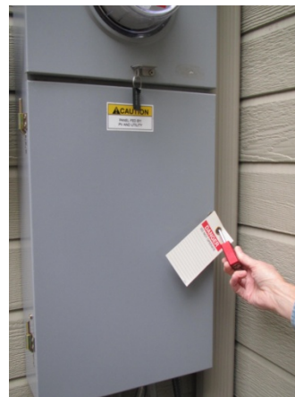
Figure 15. Lock out the electricity panel and verify that the circuit is de-energized
