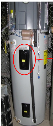
Figure 5. The Rheem HPWH with heater covers shown.
