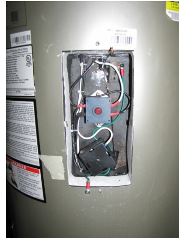
Figure 10. After the insulation is removed, the tank wall is accessible for installing a TC.
