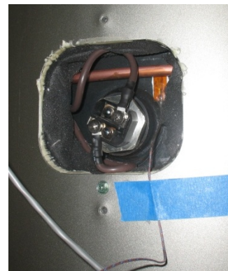
Figure 20. Surface-mounted TC at the lower tank surface
