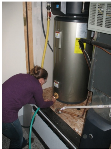
Figure 16. Connecting the hose to the drain in preparation for installing the flow meter
