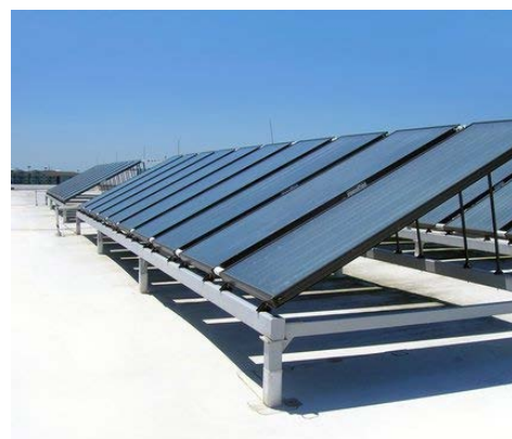
Figure 5. Commercial SWH system – IKEA Orlando
