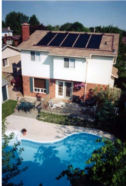
Figure C-1. Photo of polymer solar pool collectors. Photo from Aquatherm Industries, NREL/PIX 07175
