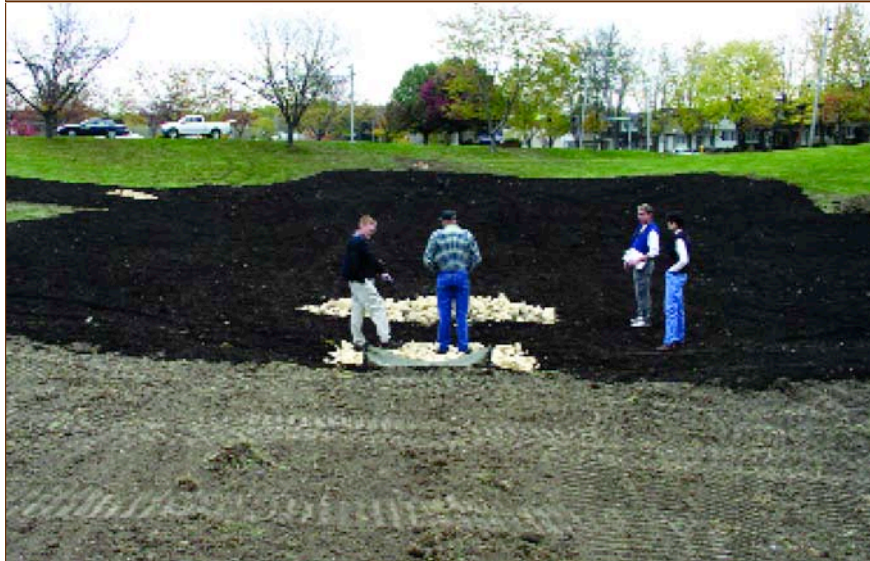
A compost blanket protects against erosion until vegetation is established on this storm water detention basin retrofit project at North High School in Davenport, Iowa. The darker color of the compost is due to its high organic matter content.
