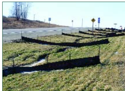
A series of silt fence ditch checks. Note how concentrated flows have caused gullying between the checks. A rolled erosion control product is recommended to enhance the effectiveness of silt fence checks.
