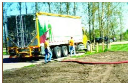
Pneumatic blower trucks are a new tool for compost-based erosion control practices.
