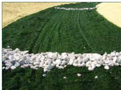
These rock check dams complement RECP's and trap sediment in concentrated flows.
