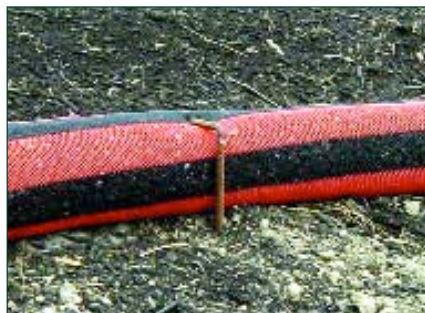
Stakes should be installed to hold compost socks in place to prevent movement.
