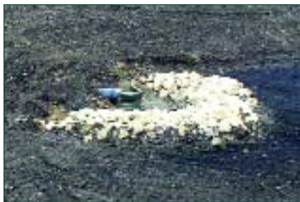
A rock check dam serves as an inlet protection device on this site.
