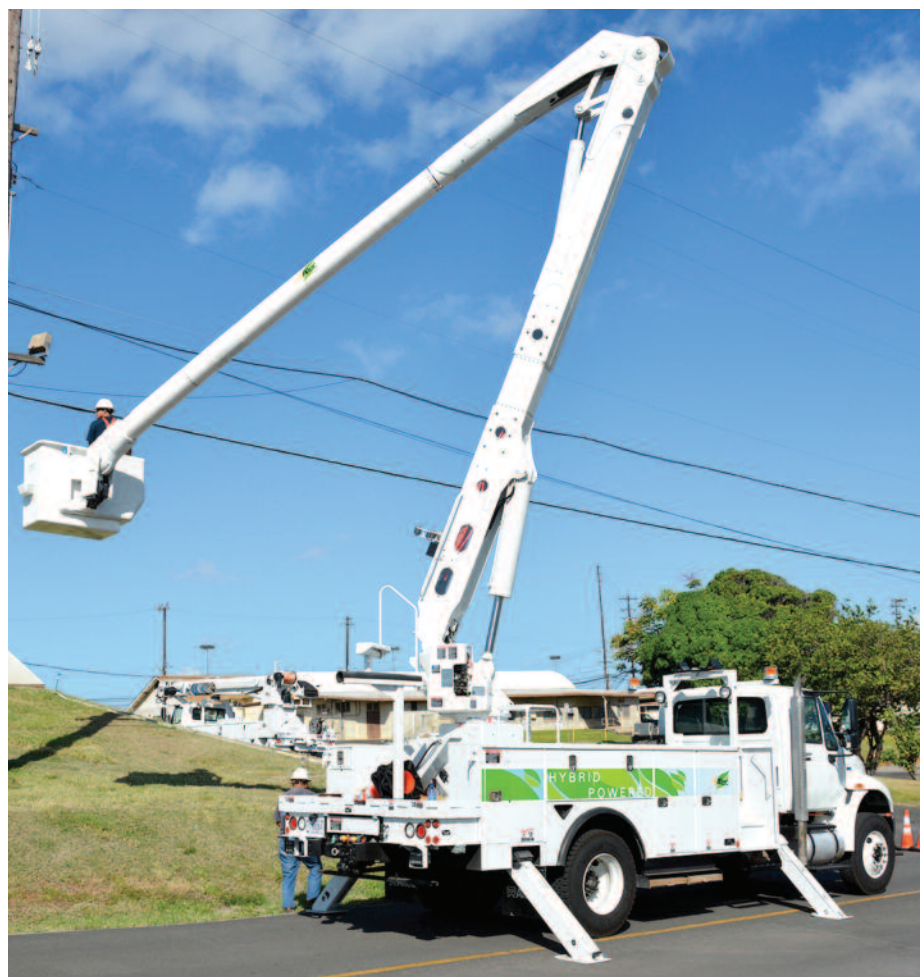
Naval Facilities Engineering Command (NAVFAC) Hawaii utilities personnel use the new hybrid bucket truck in the field for the first time. Power lines between multiple poles on the command's main compound were replaced at Joint Base Pearl Harbor-Hickam.
