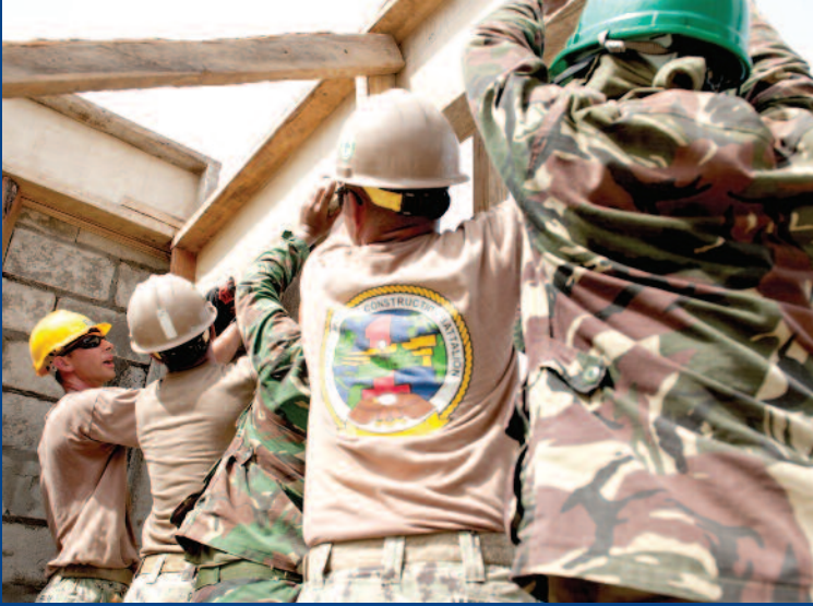
(Left) Philippine Army Corps of Engineers and U. S. Navy Seabees lift a form in place during a Pacific Partnership engineering project at San Fernando Elementary School, Tacloban, Philippines.
