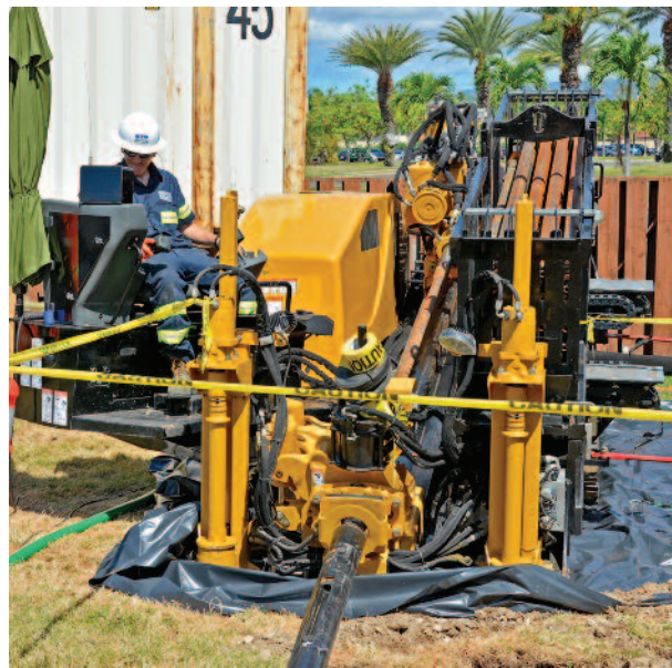
An employee from contractor AECOM operates a horizontal drill rig June 10 that will install a soil vapor extraction (SVE) system at Onizuka Village housing at Joint Base Pearl Harbor-Hickam.
