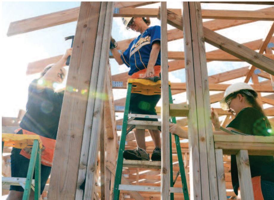
From left: Staff Sgt. Angela Parker, Maj. Amanda Evans, 15th Comptroller commander, and Staff Sgt. Nichole Rush work on the wood frame of a house while volunteering with a group of Airmen at a Honolulu Habitat for Humanity project in Waimanalo on Jan. 15.
