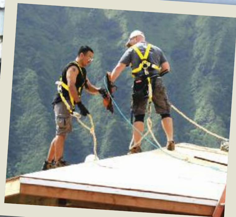
Tech. Sgt. Manny Garibay, 15th Maintenance Group, and Master Sgt. David Fritz, 65th Airlift Squadron, help build a rooftop.
