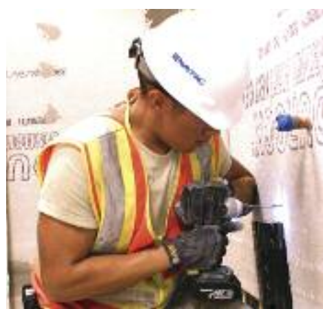
As part of the Hickam Gymnasium's foyer bathrooms complete makeover, an Air Force apprentice installs cement backer board to the walls of the men's restroom at Joint Base Pearl Harbor-Hickam.
