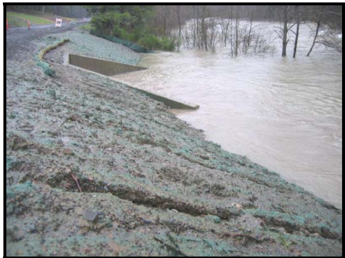
Photograph 2. Lower Mad Road (insloped and paved) looking east during December 2005 flood event. Surface runoff from road causing gully erosion on road fill and directly delivering sediment to the Mad River. Note silt fence completely inundated in background.
