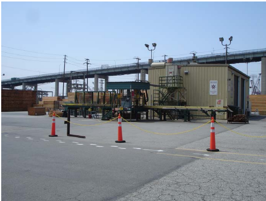
Photo 2: Saw cutting operations. Housekeeping was observed to be good in this area.
