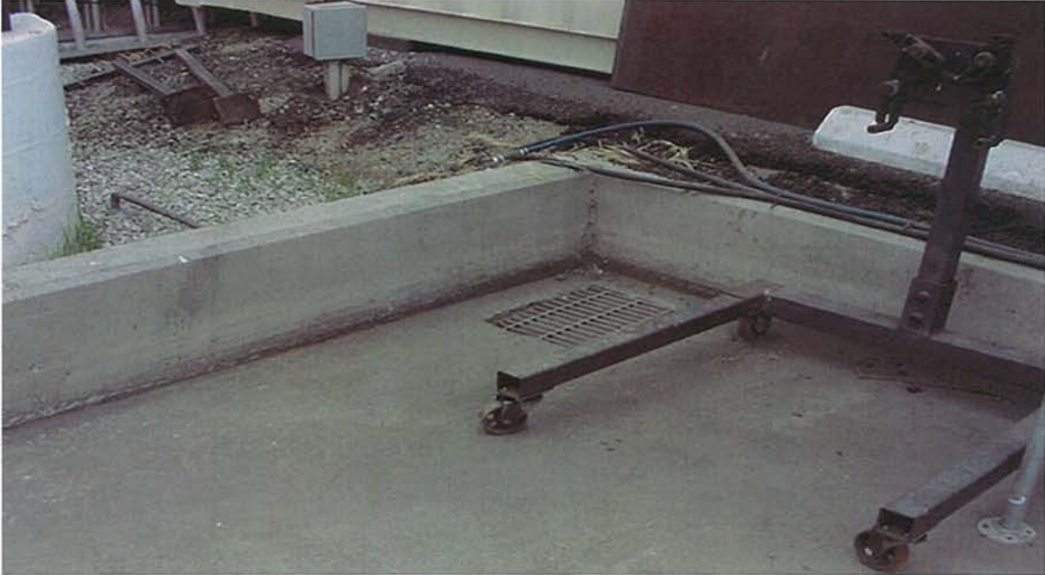
3. A closed-off sump near washing rack filled w/ dark water is not identified on the map.
