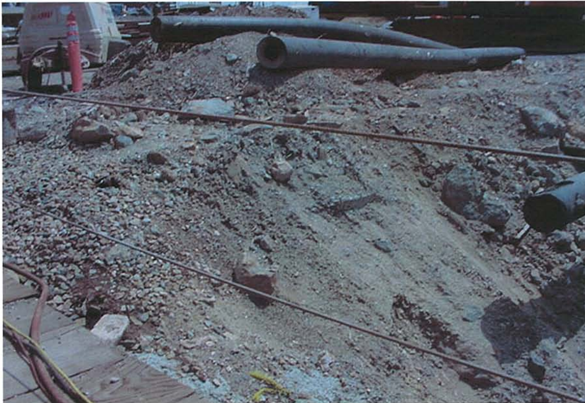
4. A mixture of sand and aggregates pile transferred from the rock barge is noted immediately adjacent to channel. The pile needs to be removed and soil erosion control should be strengthened in this nor dock area.
