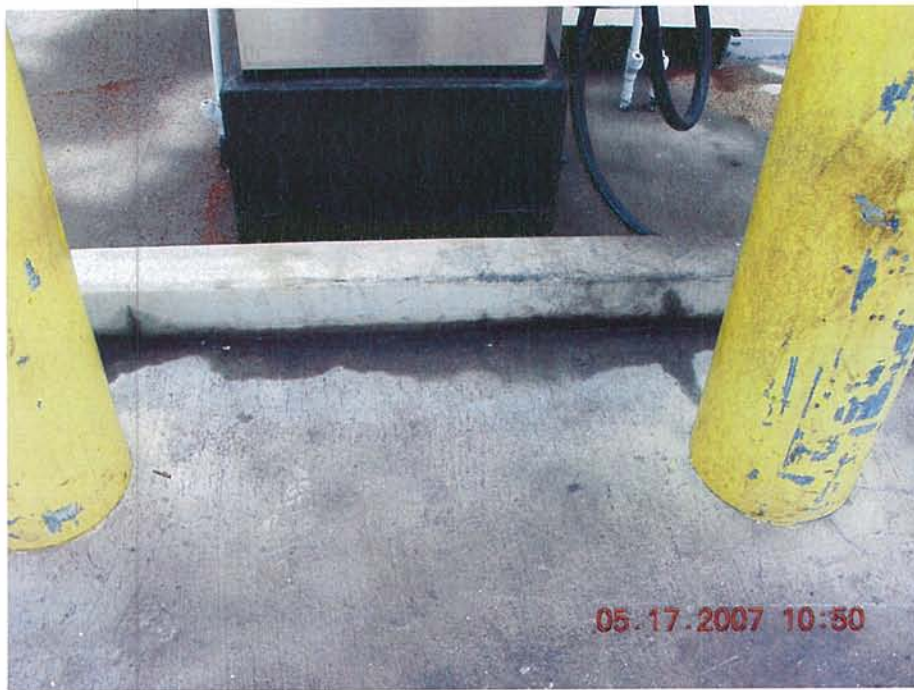
DCN0457 – Cracked and seeping secondary containment dike at west side of fuel island.
