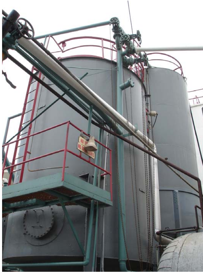
Photo 4: Tanks used to collect boiler blowdown, water softener discharges, condensate from internal heating coils and storm water.
