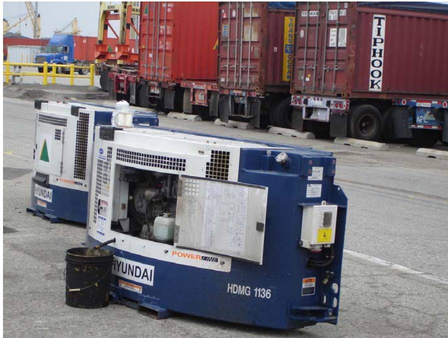
Photo 7: Maintenance (an oil change) on a refrigeration unit at an exposed uncontained area adjacent to the wash rack.
