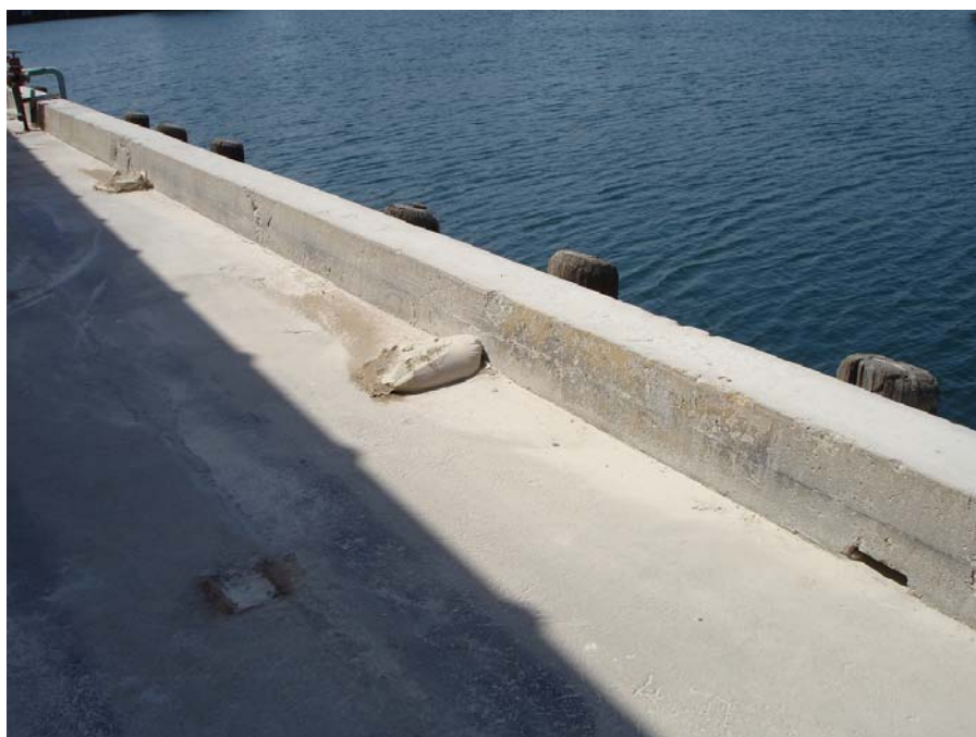
Photo 9: Open drain to receiving water at ship unloading dock, and other drains with broken sand bags.
