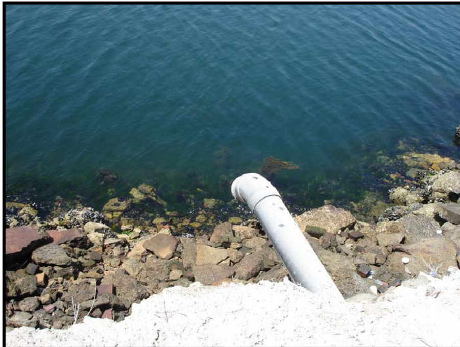
Photo 7: Location of storm water discharge to Channel Three from sump shown in Photo 6. Note the gypsum pile extends nearly into Channel Three.
