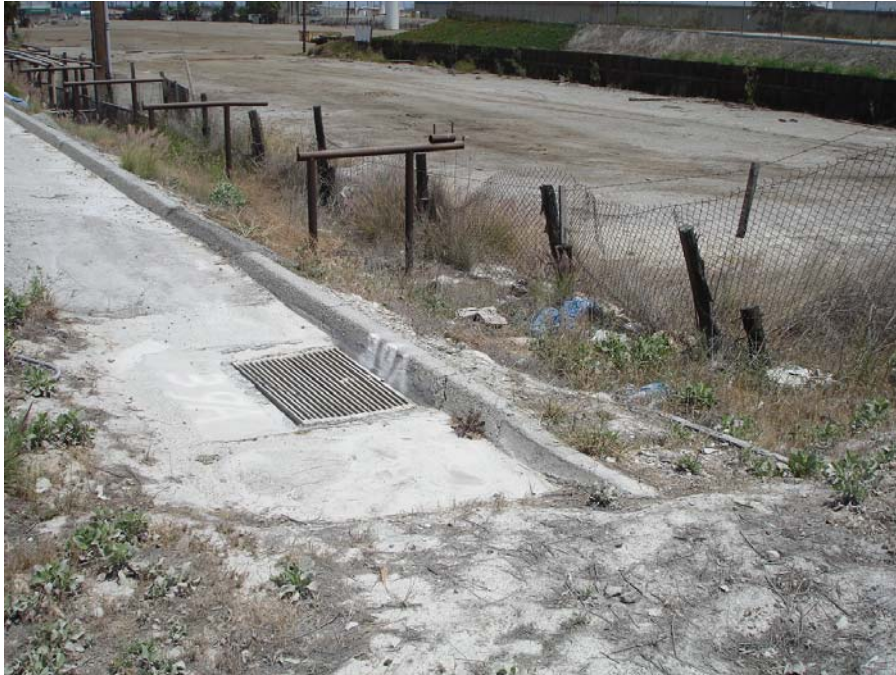
Photo 5: Evidence of gypsum powder at the storm drain southeast of the gypsum pile. This location is identified as Outfall 003 on the facility's site map.
