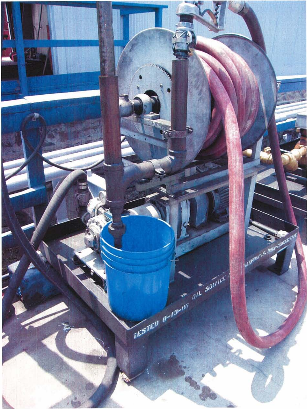
Photo 9: Fueling pump at the Fuel Loading Dock, note stains on pavement, area drains directly
