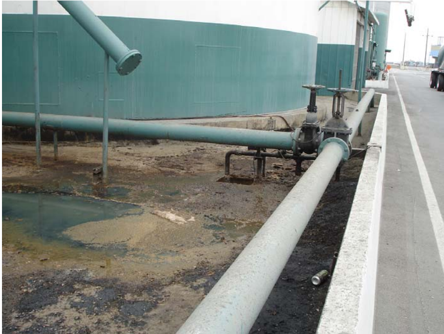
Photo 5: Oily condensate in bermed area from internal tank heating coils.
