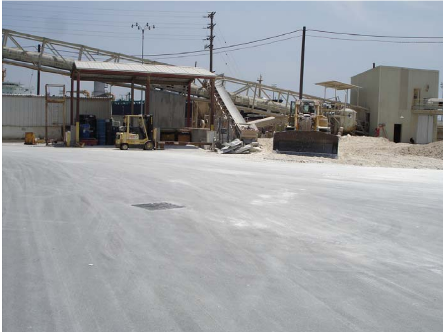
Photo 6: Storm drain east of the Tape Joint building, with exposed gypsum material in the background.
