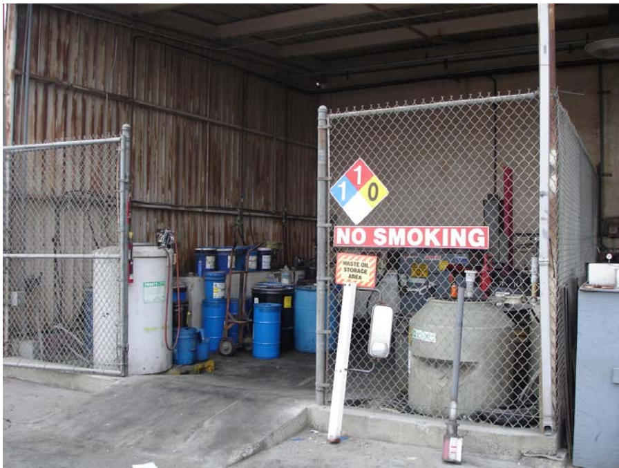
Photo 4: Cover and secondary containment were provided for waste oil and hazardous waste at the Power Shop.
