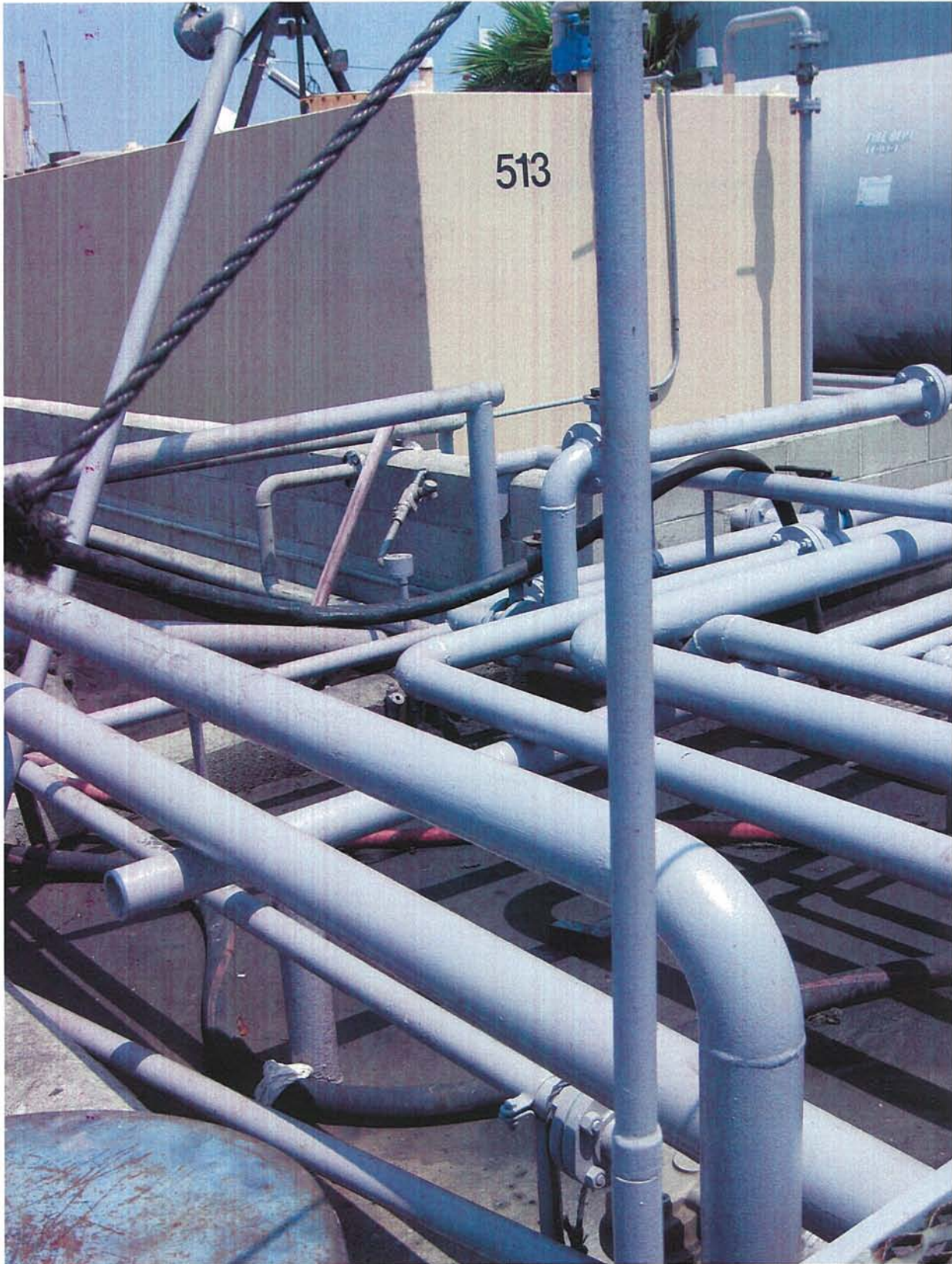
Photo 2: Stained concrete inside secondary containment area for fuel storage tanks, this area drains to a sump to be taken off-site for disposal.
