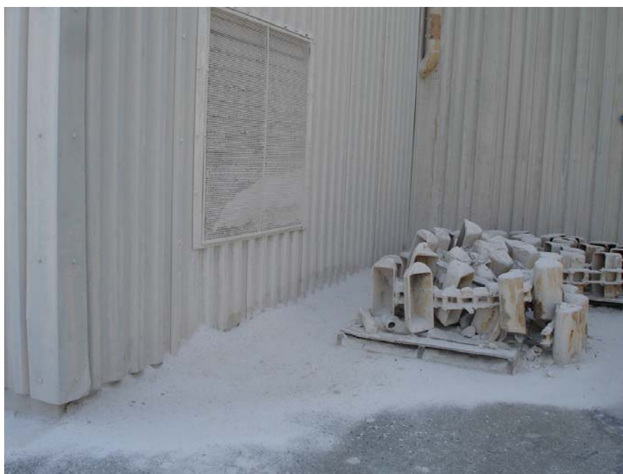
Photo 8: Gypsum powder on the ground near the Calcidyne Enclosure.
