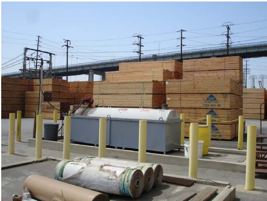
Photo 4: Diesel fuel tank with secondary containment.
