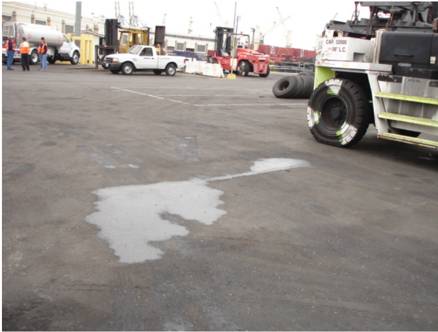
Photo 8: Exposed oil leak adjacent to maintenance shop.
