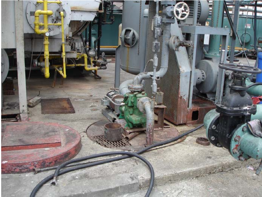
Photo 3: One of three sumps within tank farm pumped to the wastewater / storm water holding tanks.
