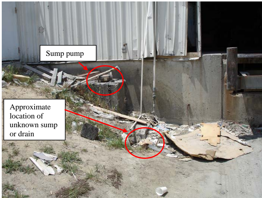
Photo 10: Poor housekeeping and out-of-service sump pump at Tape Joint Building truck dock adjacent to tanks pictured above.
