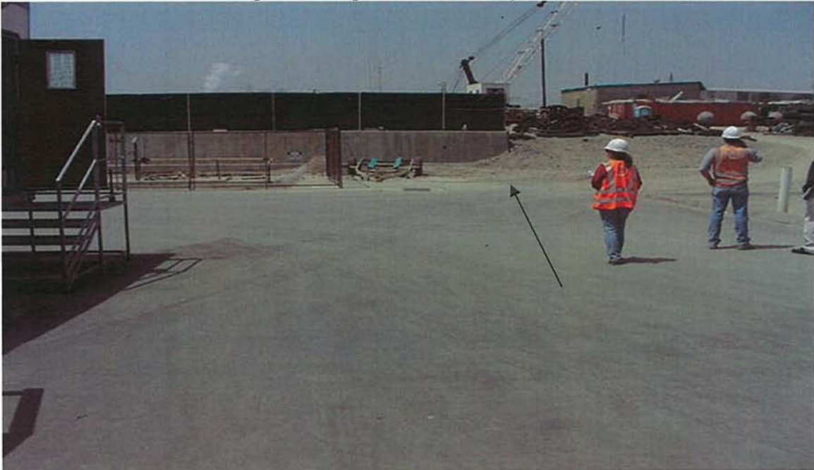
1. Storm drains in the parking lot area discharge storm water into the channel in the western boundary of the property. Note: A mixture of sand and pit gravels is by the storm drain. The storm drain receives "D" street surface run-on and part of on-site runoff.
