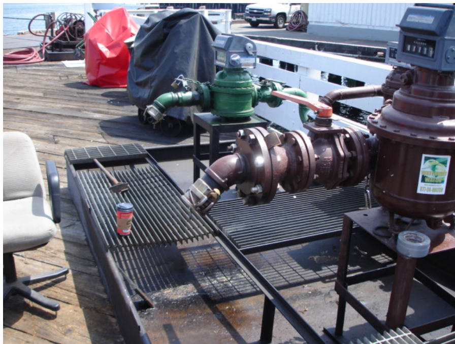
Photo 2: Oil valves at main dock with containment.
