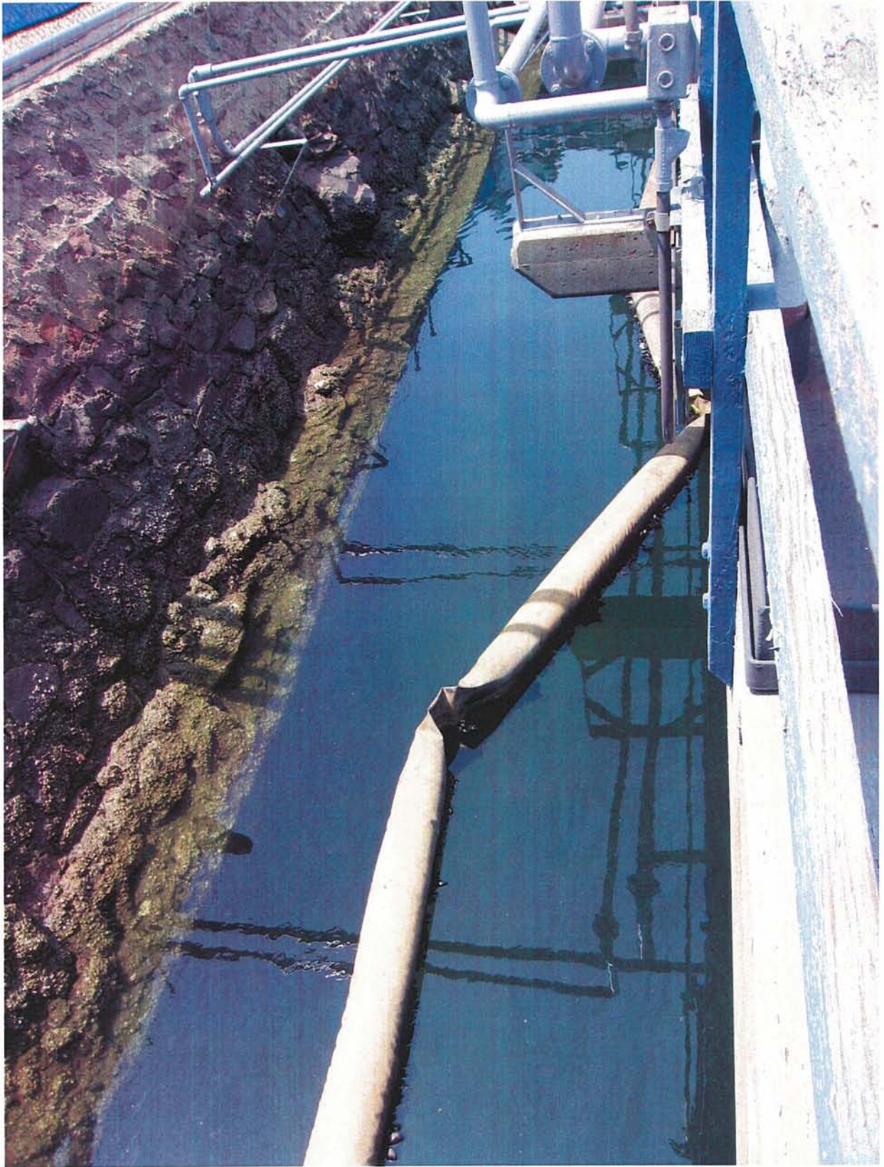
Photo 15: Permanent boom behind the Fuel Dock, note oily sheen.
