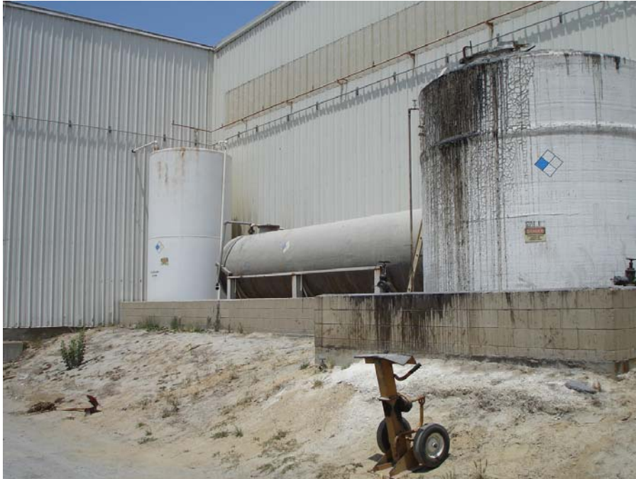
Photo 9: Evidence of spillage from tank near Tape Joint Building truck dock.
