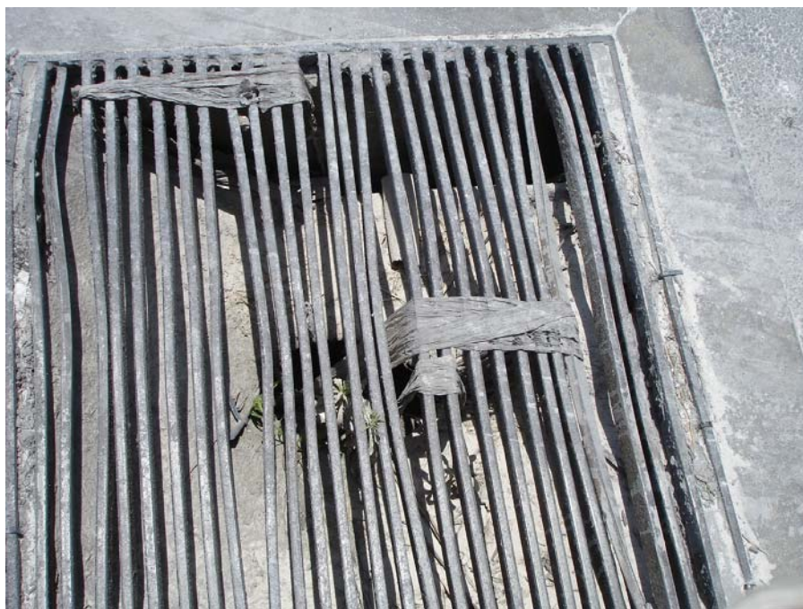
Photo 7: Close-up of drain pictured above.
