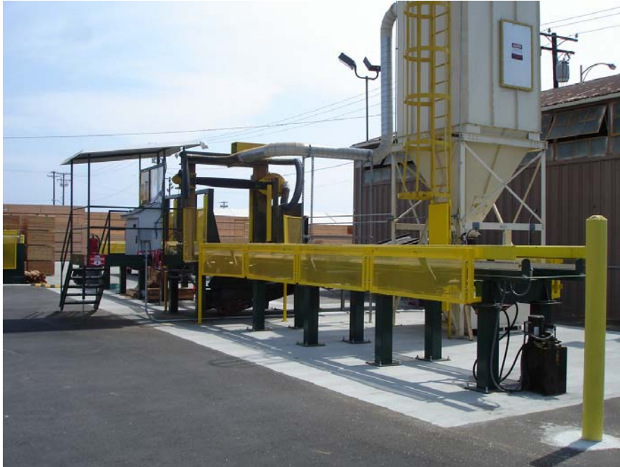
Photo 3: Saw cutting operations. Housekeeping was observed to be good in this area.
