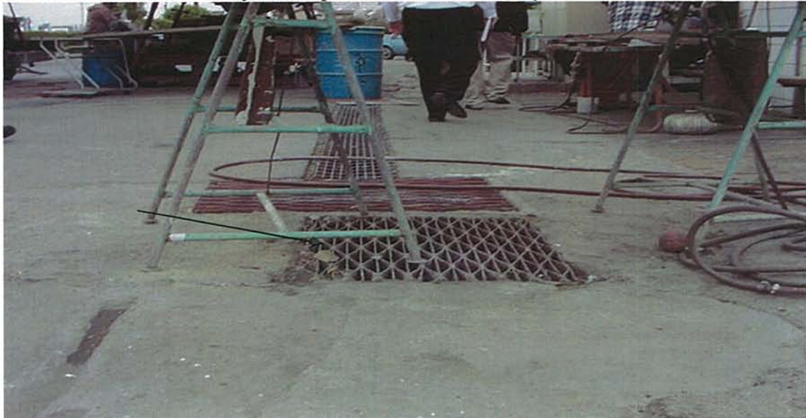
2. Wastewater collection trough connected to the treatment system in the boat repair and dry-dock storage yard.
