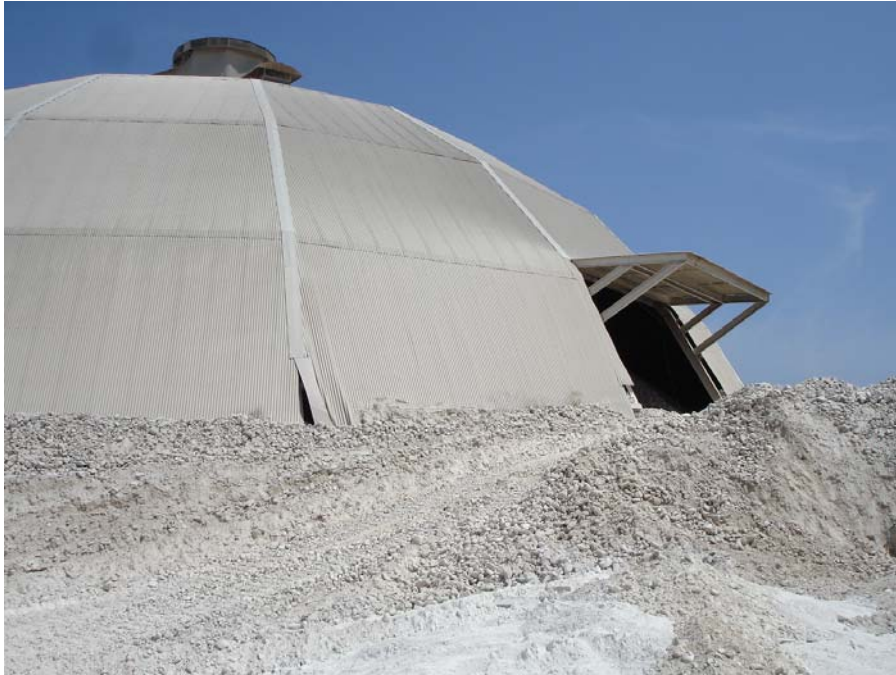
Photo 3: Gypsum rock dome and exposed gypsum material and associated fines on the northwest side of the facility.
