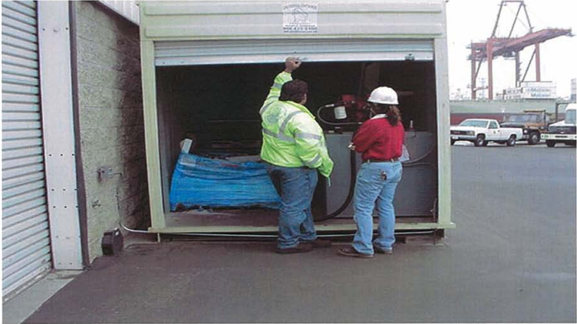
5. Fueling tank is located inside the container. Spill may occur during fuel transferring. Source control is recommended to be implemented during fuel transferring.
