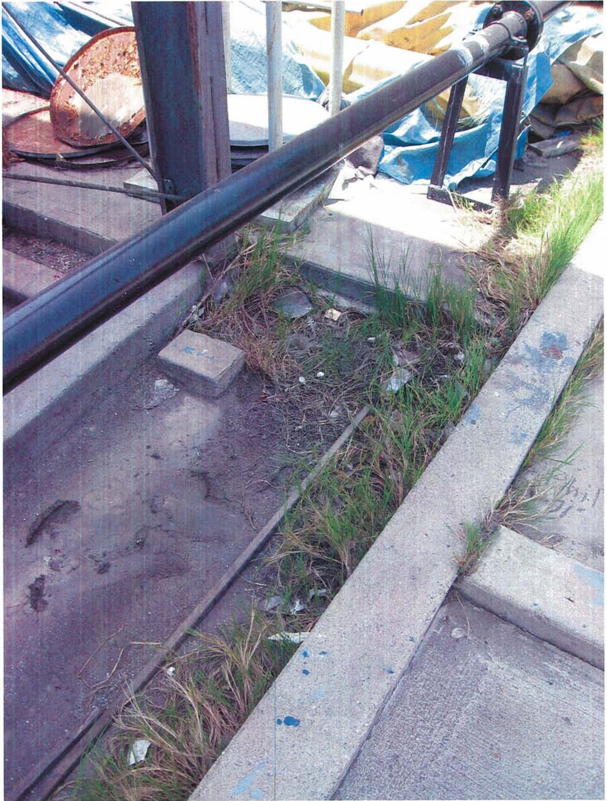
Photo 8: Photo of the end of the berm around area shown in Photo 7.
