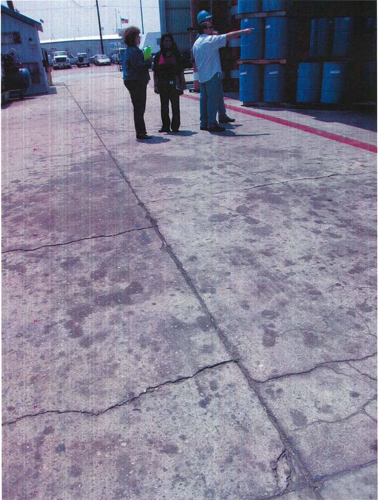
Photo 6: Note staining on pavement, this area also drains toward off-site storm drains that lead to the Harbor, (covered Storage Area to the right).
