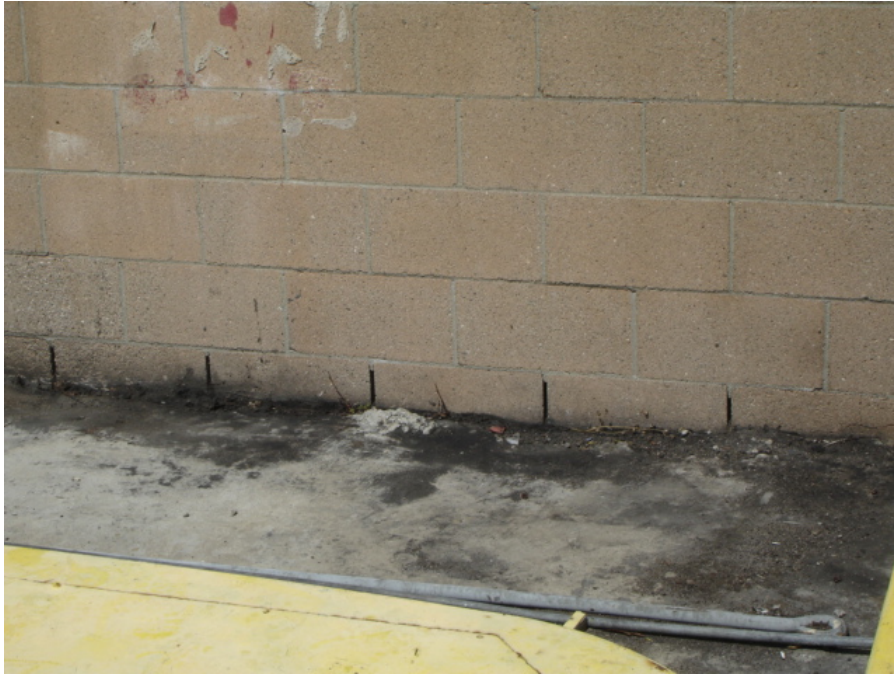
Photo 9: Mortar missing from block wall at in-ground containment vault. Rip-rap and the Harbor are located on the other side of the wall.
