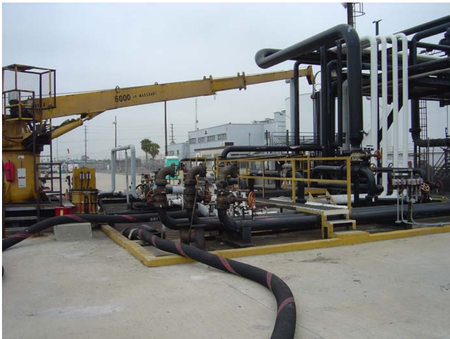
Photo 2: The loading/unloading area (pipeline manifolds and bunkering lines) is enclosed within “dock pans” which discharge to a holding tank.
