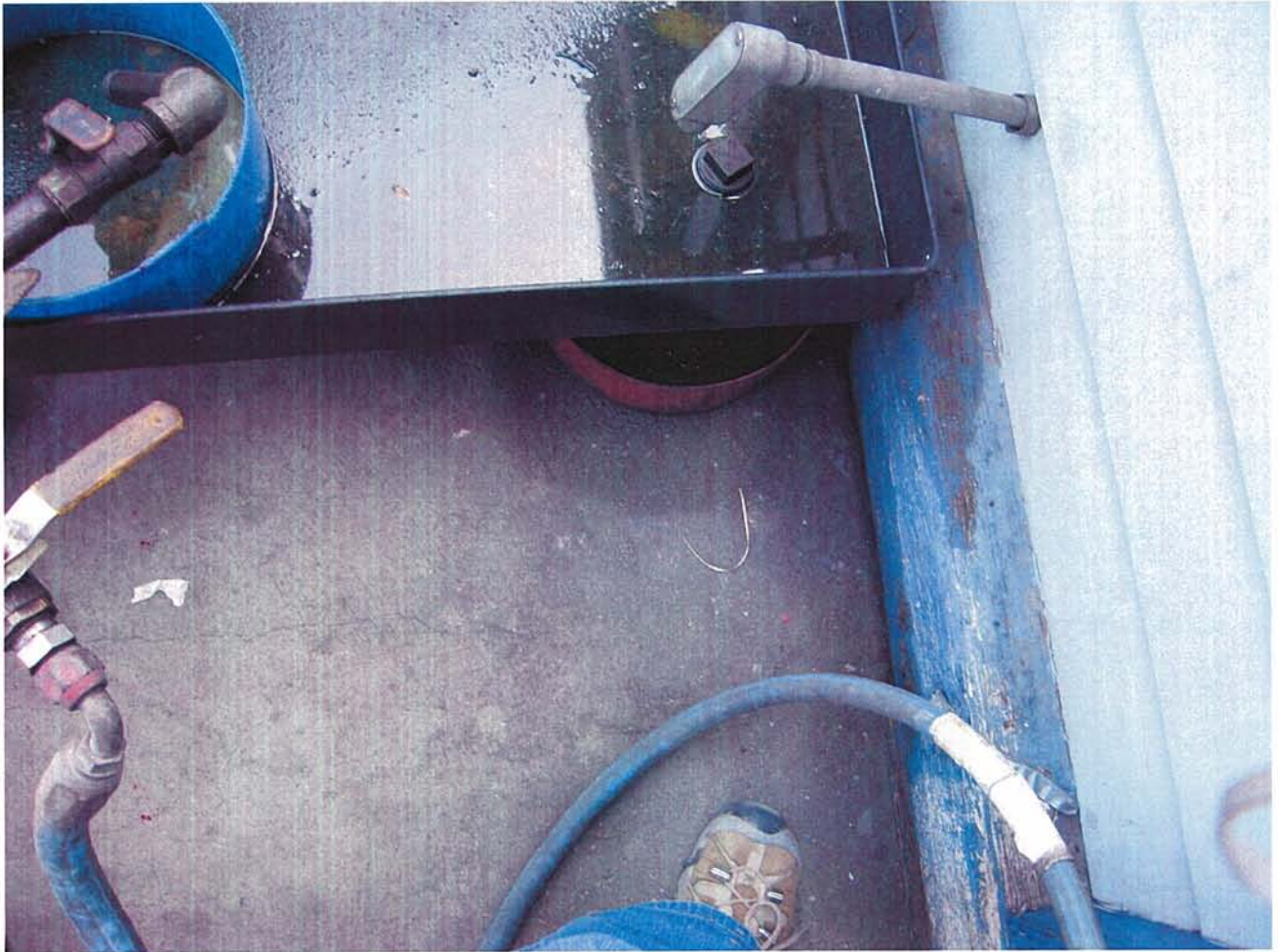
Photo 16: Drain plug in the secondary containment unit for the fuel pumps, with a container below. The concrete is stained around the container.
