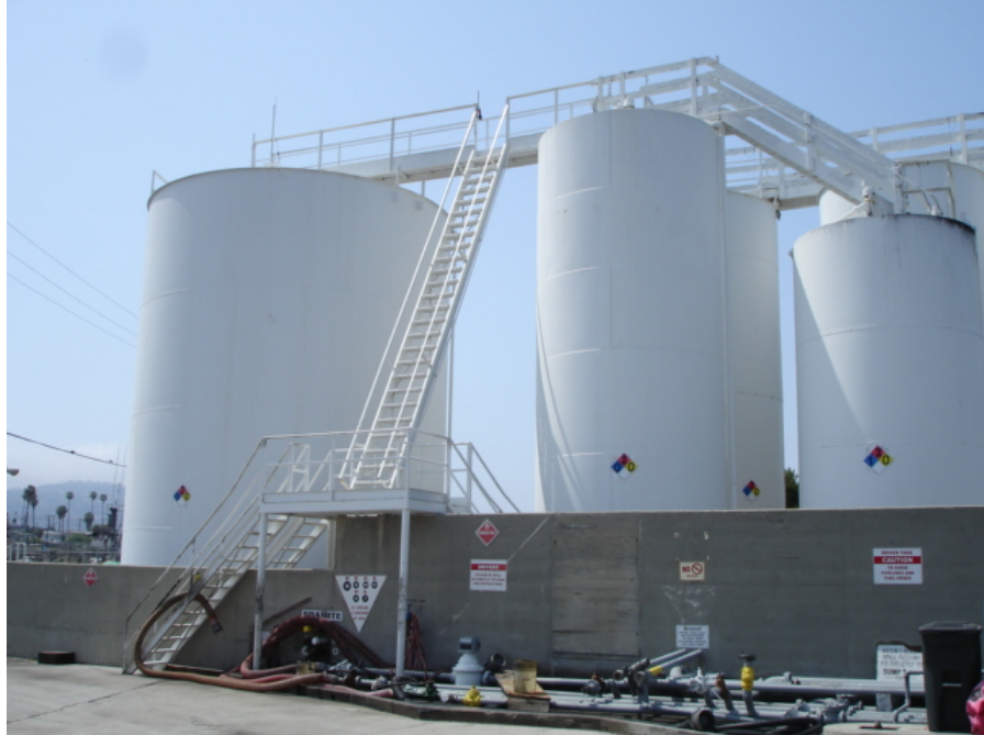
Photo 6: Bulk petroleum storage tanks.
