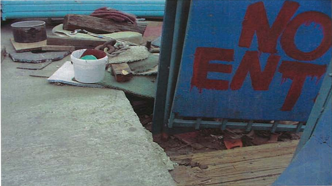
3. Some lifting equipment and accumulated debris was noted by the crane.
