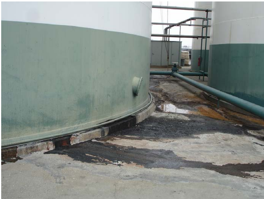
Photo 6: Apparent leak from bulk oil storage tank and oily condensate from internal heating coils.
