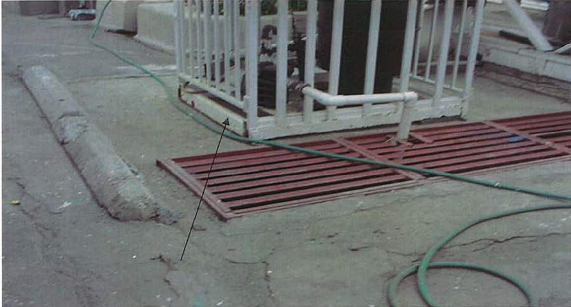
1. Wastewater Treatment System is permitted under LA City Industrial Waste Unit.
