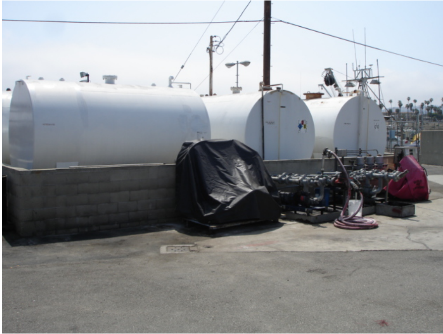
Photo 7: Bulk petroleum storage tanks and drain leading to in-ground containment vault.
