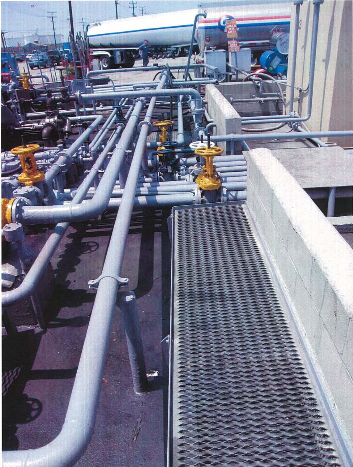
Photo 4: Stained concrete inside secondary containment area for fuel storage tanks, this area drains to a sump to be taken off-site for disposal.
