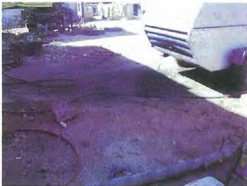
Photo 52: Staining of the ground by exhaust from an on-site air compressor.
