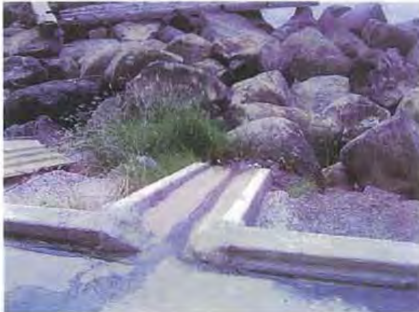
Photo 24: Another photograph of the storm water outfall for the area behind the metal working building. Wash water runoff is visible discharging down the outfall.
