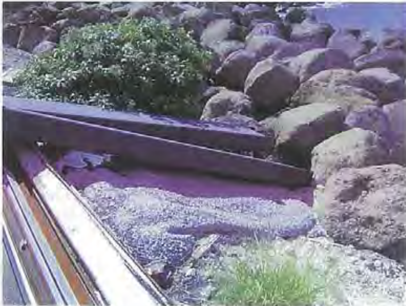
Photo 22: Evidence of concrete spillage from an on-site construction activity (possibly the construction of the concreted area itself or the berm) toward the receiving water. It is unclear if any of the concrete actually entered the receiving water. However this photo demonstrates a lack of effective best management practices utilized for the construction project by the Discharger this close to the edge of the receiving water.
