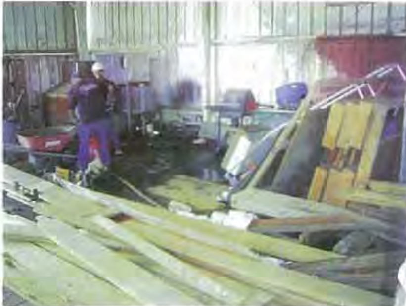
Photo 37: Two workers were observed mixing cement on the work barge. Wet cement was observed on the ground of the work barge. Runoff from the cement mixing was observed running under the wall and down the side of the work barge into the receiving water, as shown in Photo No. 39.
