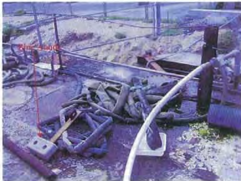
Photo 43: These water lines are used to supply the workers with potable water as they work on-board vessels. The line/hose hook ups were observed leaking and draining over the edge of the work barge. Also pictured above is a zinc anode on the deck of the work barge, near the draining water.
