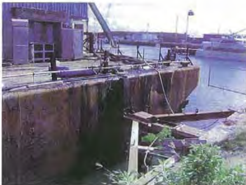
Photo 44: Potable water from hoses on the work barge was observed flowing over the deck and into the receiving water.
