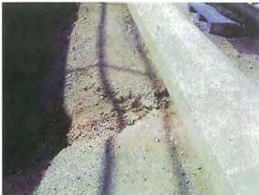
Photo 58: Another gap in the berm.
