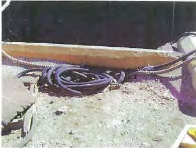
Photo 54: Another gap developed through erosion in the berm.
