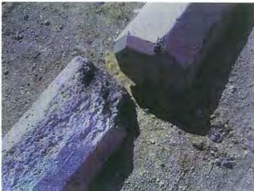
Photo 55: Another gap in the berm.
