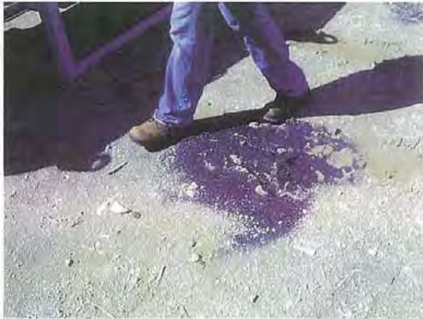
Photo 56: Sand blasting grit was observed on the ground, exposed to potential storm water runoff.
