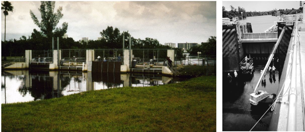
Figure 14. Water control structure retrofitted with pressure sensitive technology (left). Retrofitting of St. Lucie Lock with acoustic sensors (right) to protect manatees from being crushed as the gates close. (Photographs by FWS and B. Brooks)
