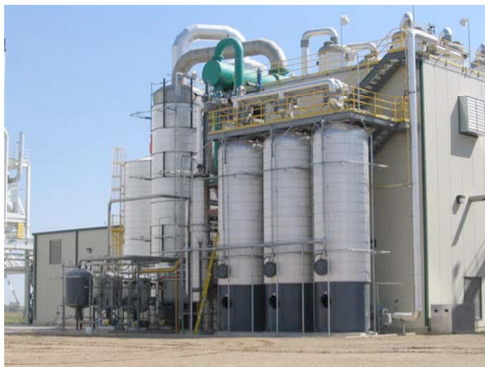
Front Range Energy's ethanol plant in Windsor, CO.
