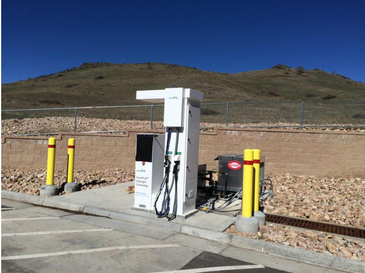
Figure 4. Hydrogen dispenser (note high- and low-pressure fueling hoses)
