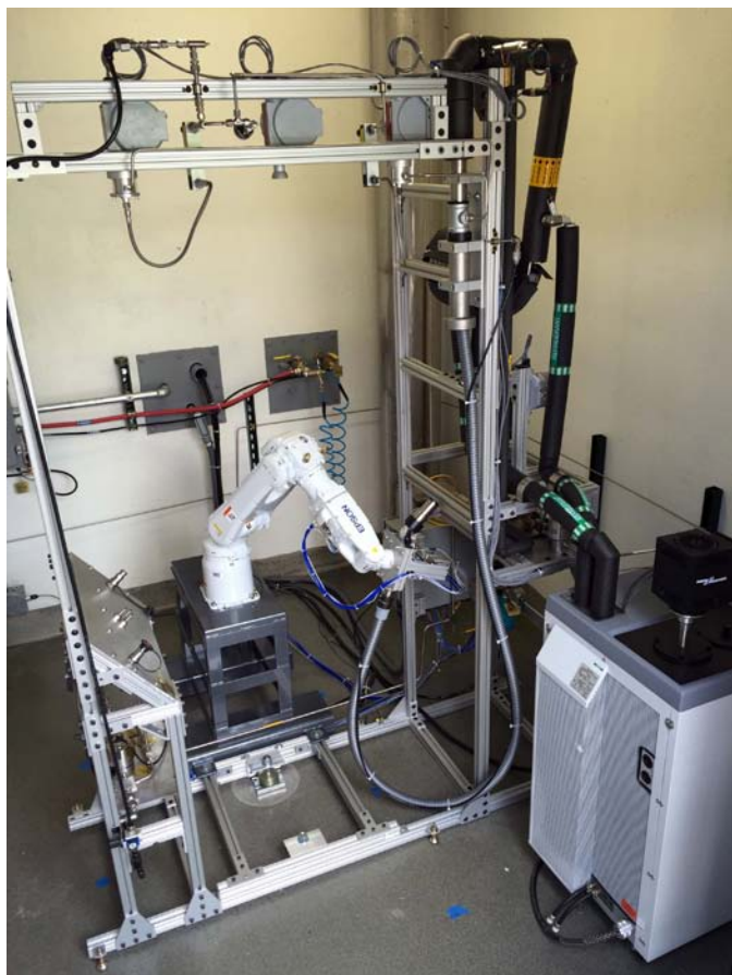
FIGURE 1. Completed hose test stand installed in HPTB
