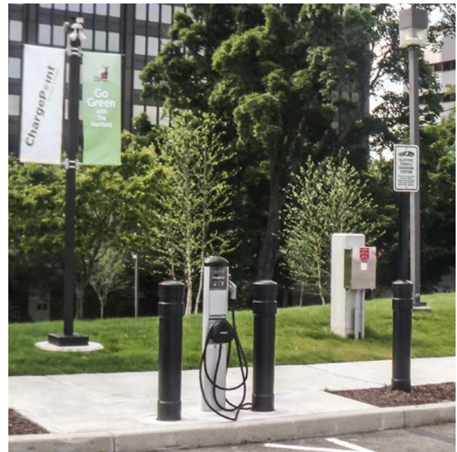
The Hartford offers workplace charging at various locations across Connecticut, helping the company make progress toward its goal of reducing greenhouse gas emissions 20% by 2017. Photo from The Hartford, NREL 26470
