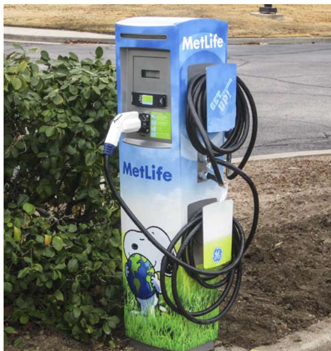
MetLife has installed PEV charging stations for employee use at 14 of its locations across the country. Photo from Josh Weiner, MetLife, NREL 26465
