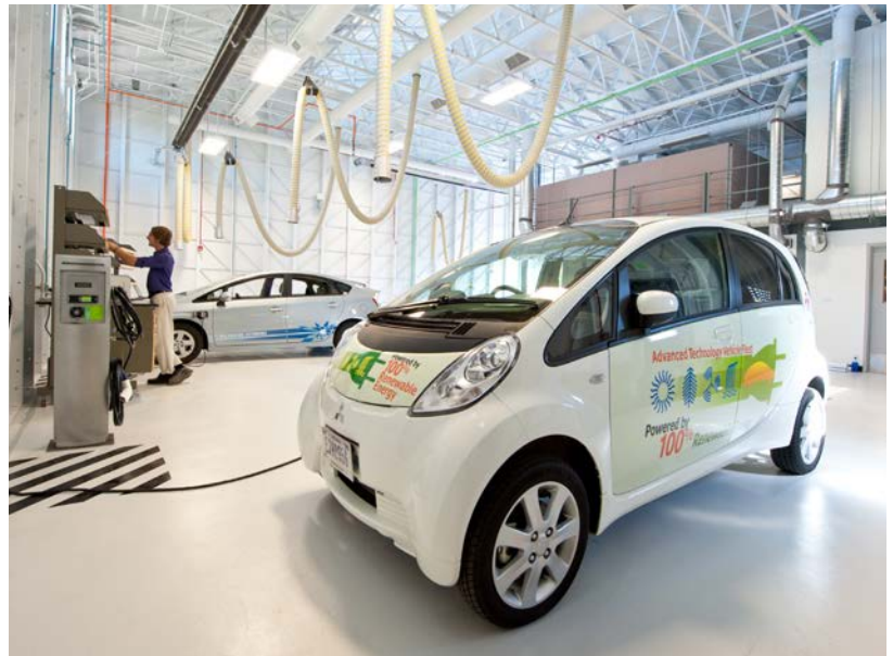
PEV charging in the VTIF. Photo by Dennis Schroeder, NREL 19758
