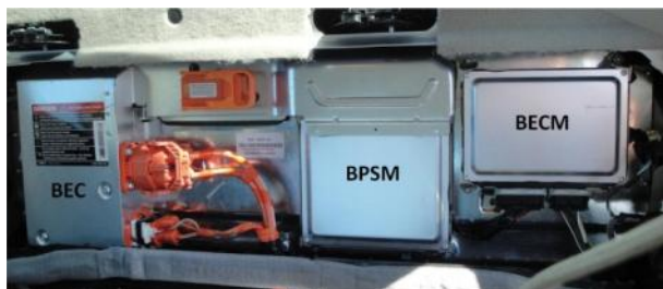
Figure 1. Photo of the Fusion Hybrid's HVTB (Photo credit: John Ireland, NREL).
