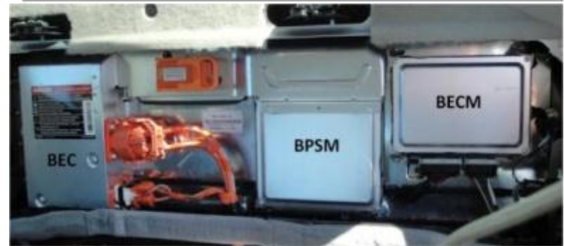
Fusion HEV test platform and traction battery with Bussed Electrical Center (BEC), Battery Pack Sensor Module (BPSM), and Battery Energy Control Module (BECM)
