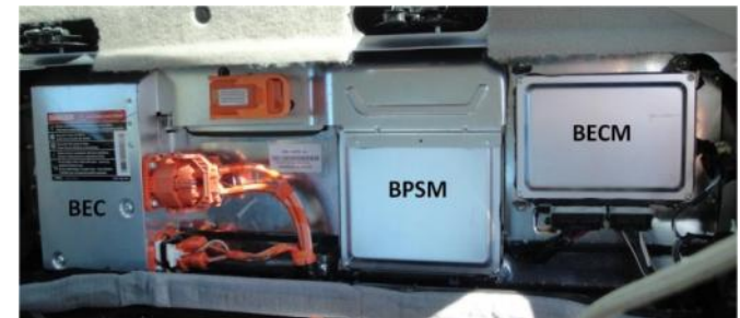
Fusion test platform and traction battery with Bussed Electrical Center (BEC), Battery Pack Sensor Module (BPSM) and Battery Energy Control Module (BECM)
