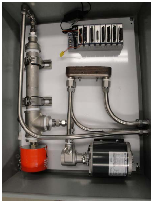
Liquid-handling thermal management in-the-loop; Photo credit: Dirk Long, NREL
