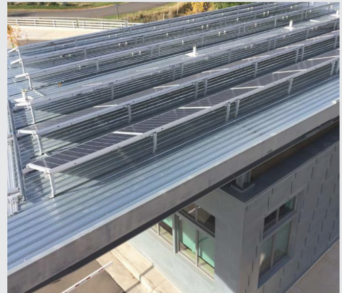
The SSEB at NREL had eleven new solar PV panels installed to bring the building back to a net zero energy status.
