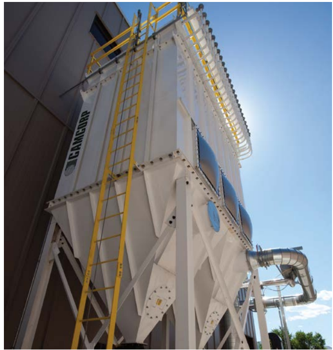
Baghouse filter at the Integrated Biorefinery Research Facility. The baghouse filter collects dust and particulates generated during the biomass milling process of biofuel production. Photo by Dennis Schroeder, NREL 17679
