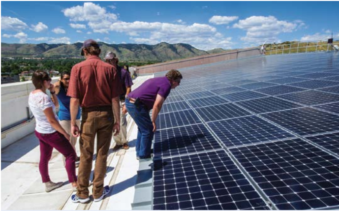
Members of the U.S. Department of Homeland Security sustainability team tour the photovoltaic array on the roof of the Research Support Facility. Photo by Dennis Schroeder, NREL 34562
