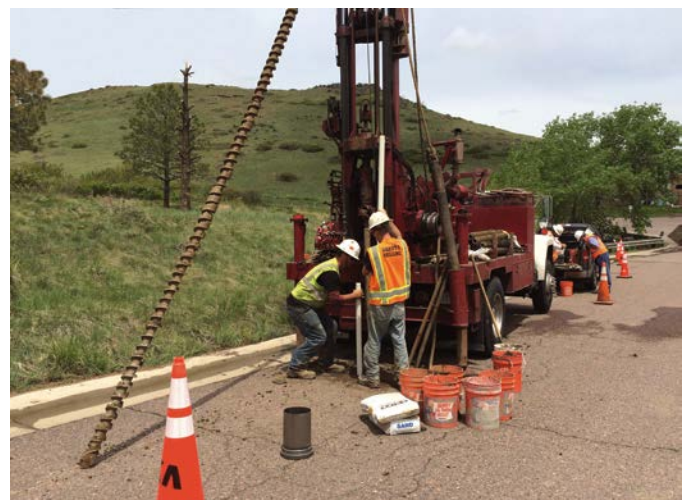
Installation of a groundwater monitoring well near the Field Testing Laboratory Building at the STM site. Photo by Genevieve Braus, NREL 36268
