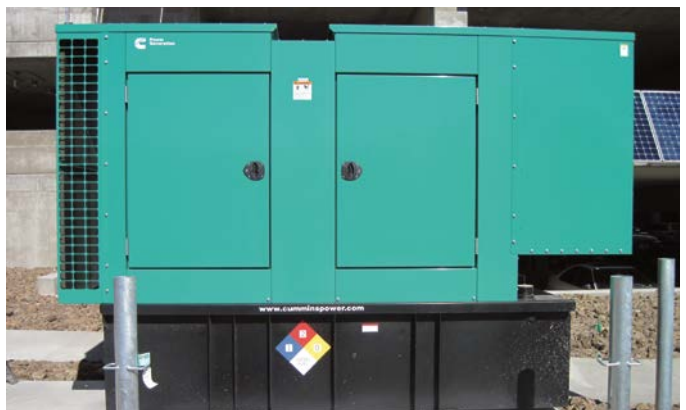
Emergency generator near the employee parking garage at the STM site. Photo by Genevieve Braus, NREL 36262
