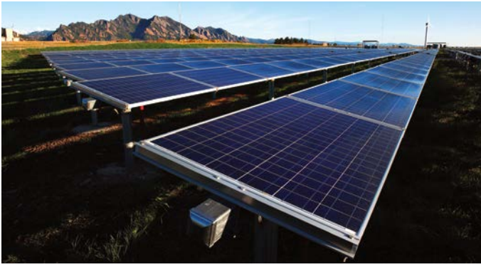
1.1MW solar photovoltaic array at the NWTC. Photo by Dennis Schroeder, NREL 31432
