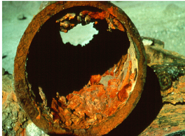
Salinity damages to municipal water pipe.
