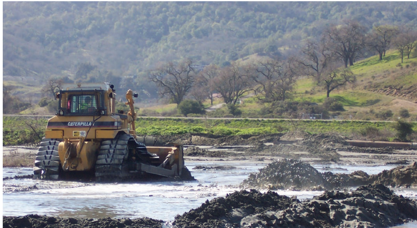
A bulldozer spreads dredged mud at the Hamilton Field wetland restoration site in Marin County, California.
