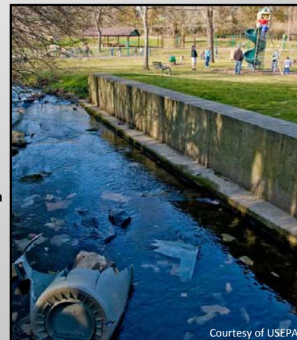
Removal of riparian vegetation and channel hardening in an urban stream
