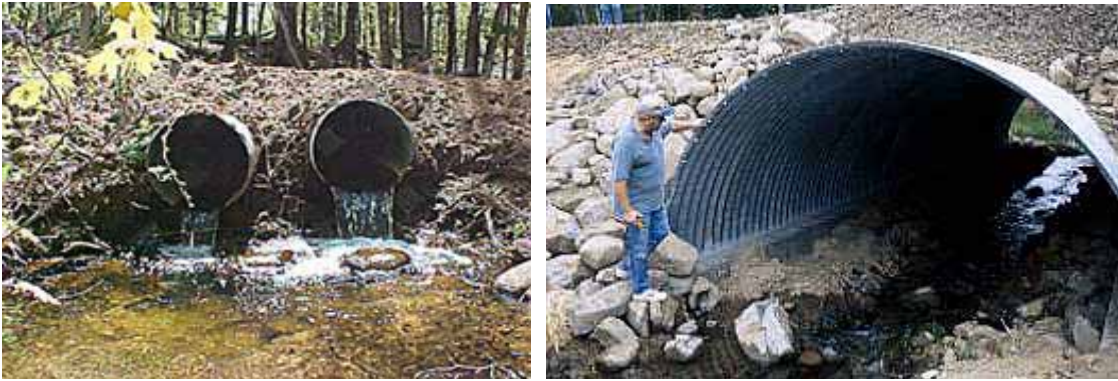
Figure 12: Perched culvert on the left prevents fish passage upstream. The culvert on the right is sized and placed properly, maintaining the connectivity of the stream. (photos: USFWS Region 3)
