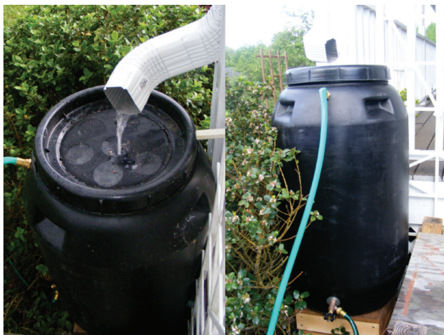
Figure 3. A rain barrel system for rainwater harvesting.
