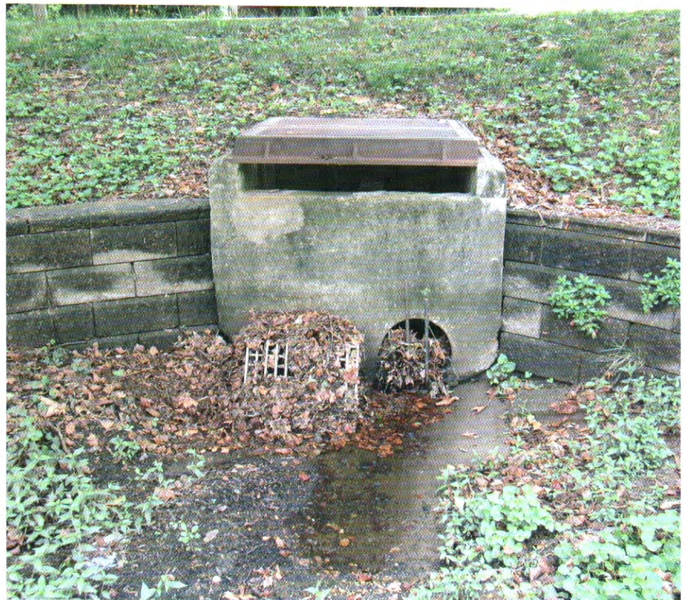
Clogged detention basin outlets lose their ability to dissipate flood waters and prevent the flooding of local properties.
