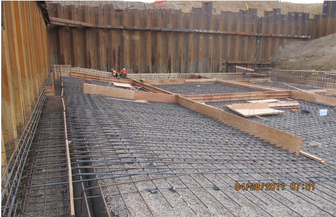
Balfour Beatty bottom mat of reinforcing steel and formwork for pumping plant slab.
