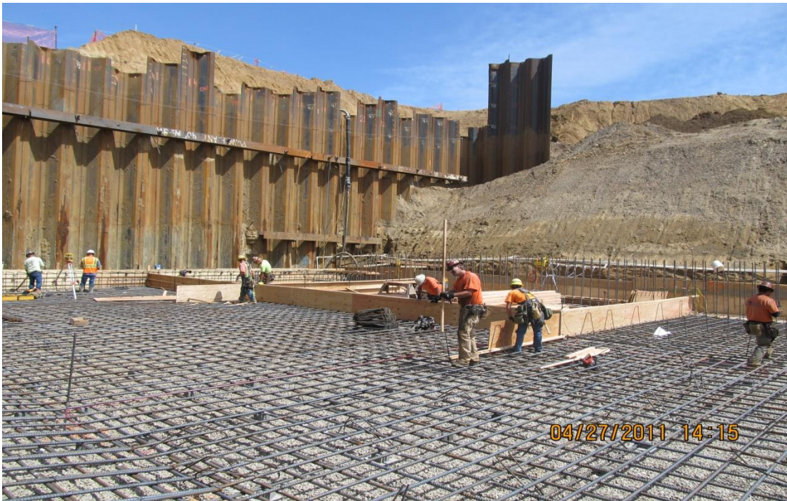
Balfour Beatty carpenter crew building forms for pumping plant intake slab concrete placements.
