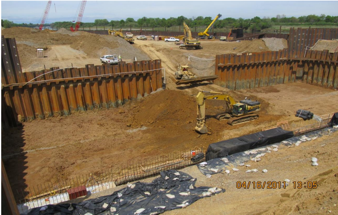
Balfour Beatty subcontractor Meyers excavating to sub grade in the pumping plant.
