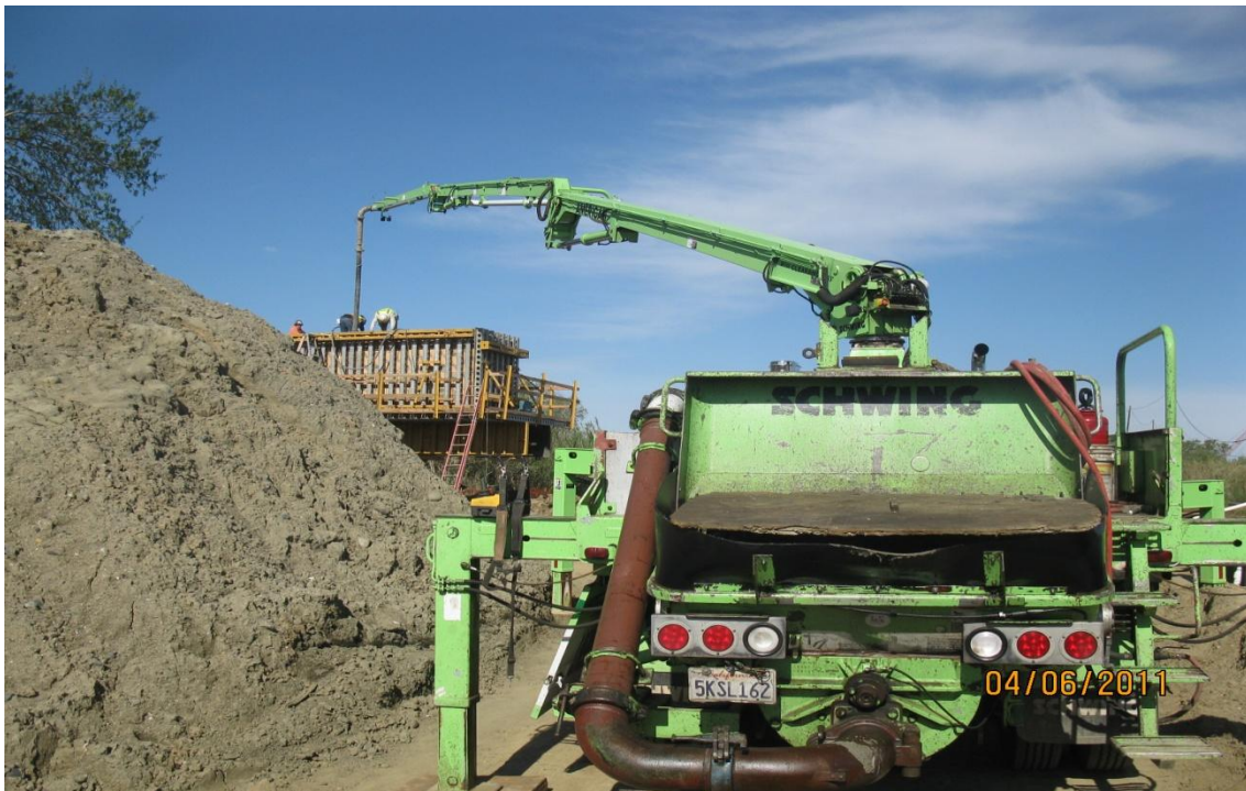
West Bay Builder's subcontractor American Concrete placing concrete in a column cap.
