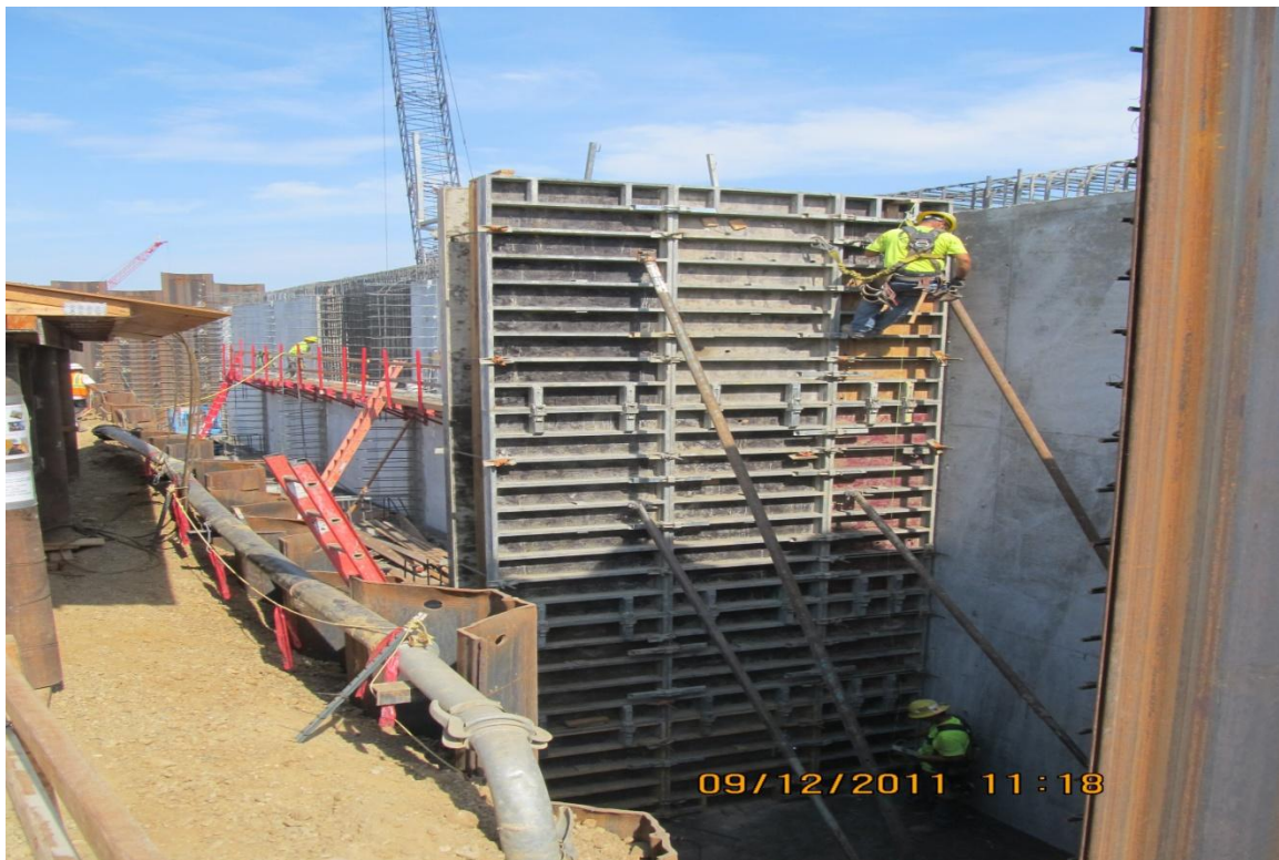
Balfour Beatty carpenter securing a buttress wall form of the pumping plant.
