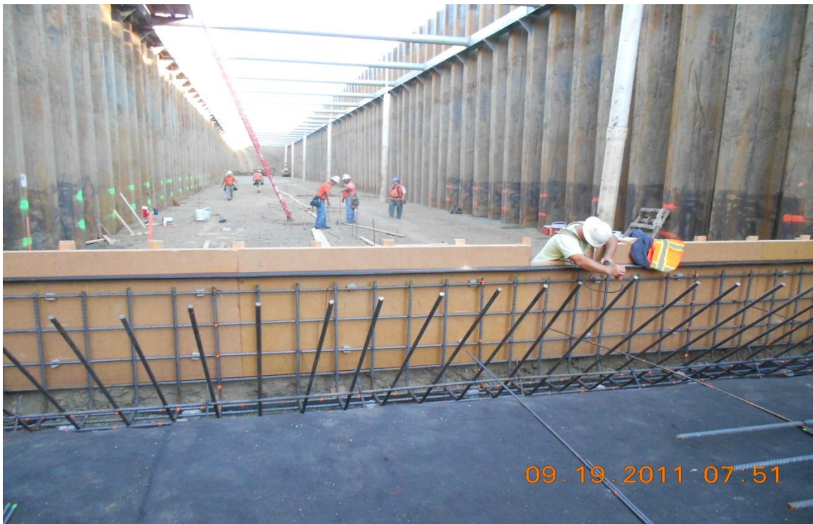
West Bay Builders carpenter working on bulkhead at beginning of siphon inlet structure.
