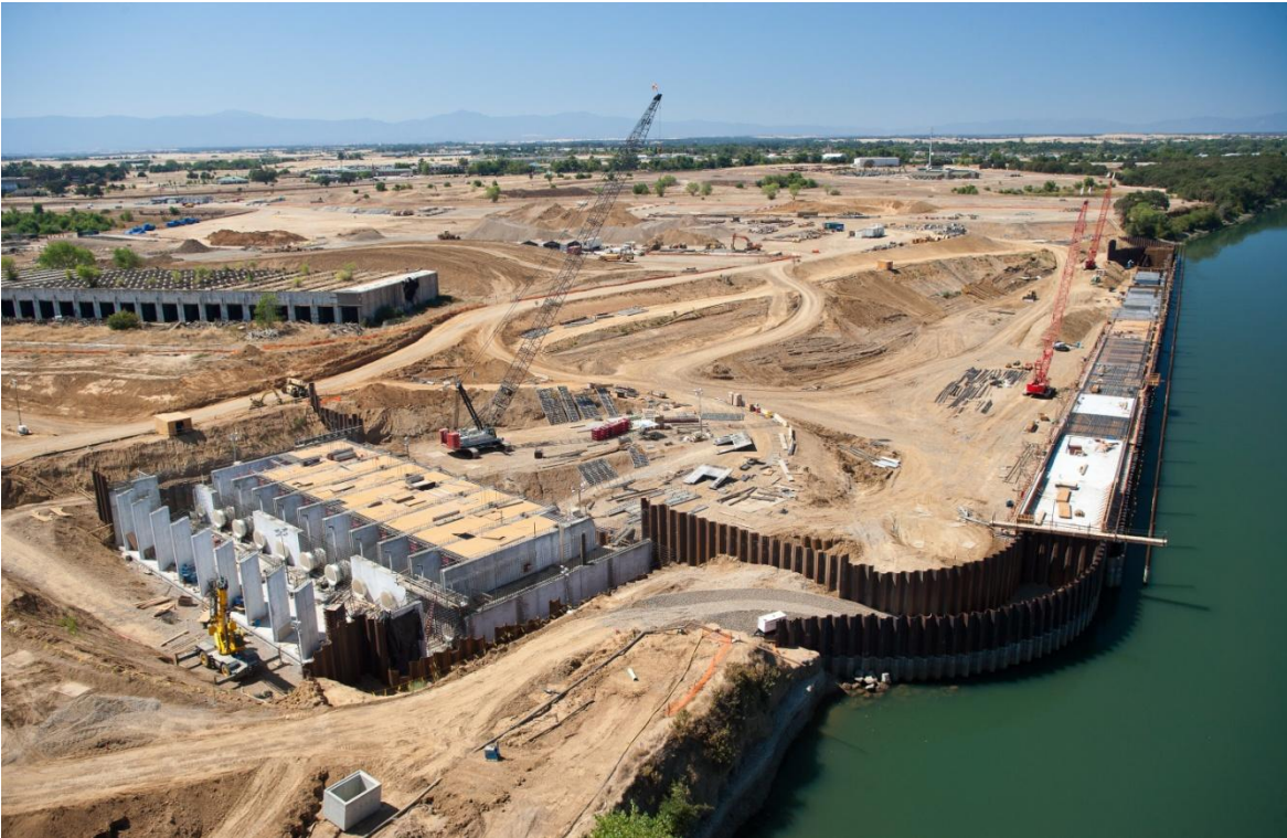
Aerial view of pumping plant and fish screen.
